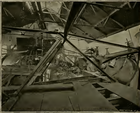
POCKET PLATING RESTING ON TOP OF BOILERS.
