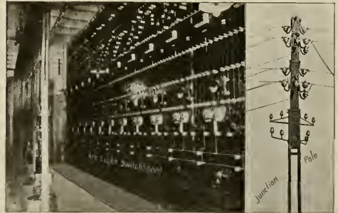
THE ROME LIGHT AND POWER STATION.
