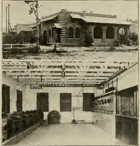
SUB-STATION IN BAKERSFIELD—INTERIOR OF TRANSFORMER AND SWITCH BOARD ROOM.
