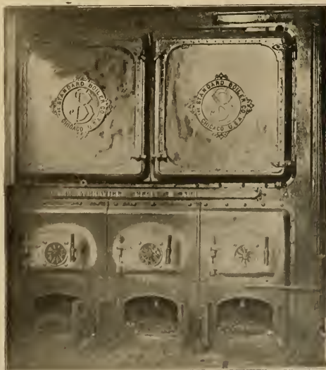
STANDARD BOILERS IN ELGIN POWER STATION.
