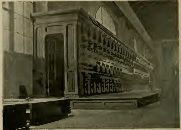
FIG. 7.—GENERAL VIEW OF SWITCHBOARD.
