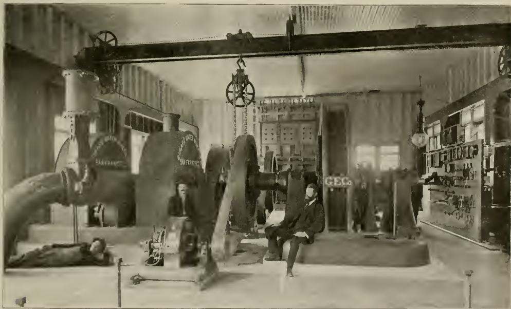
INTERIOR OF THE GENERATING STATION—POWER DEVELOPMENT COMPANY, BAKERSFIELD, CAL.
