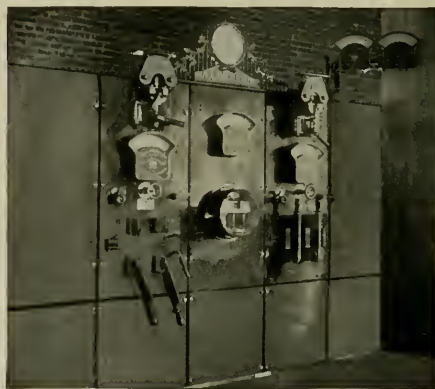
SWITCH BOARD, BERLIN POWER STATION.
