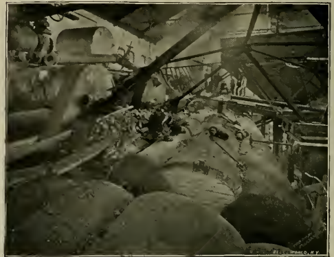
TOP OF BOILERS AND STEAM HEADER.
