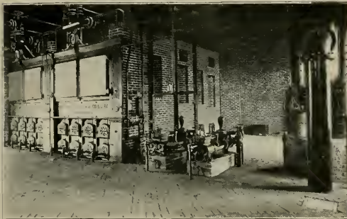
BOILER ROOM—MARION CITY EAILWAY.
