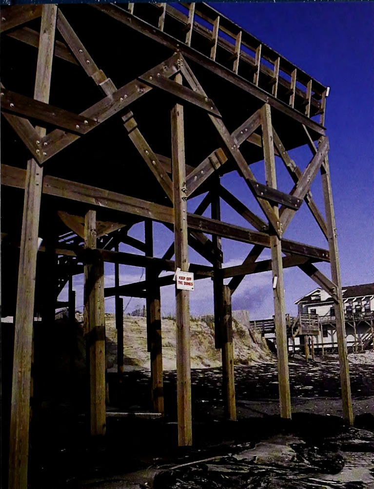
Sea Grant research led to requirements for deeper pilings to provide resistance for oceanfront homes. Photo by Spencer Rogers
