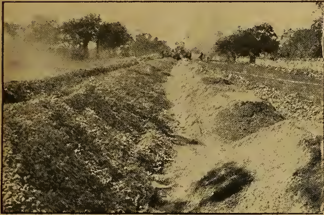
After the roadbed has been graded, sand and gravel are unloaded on it in the proportions used in mixing
