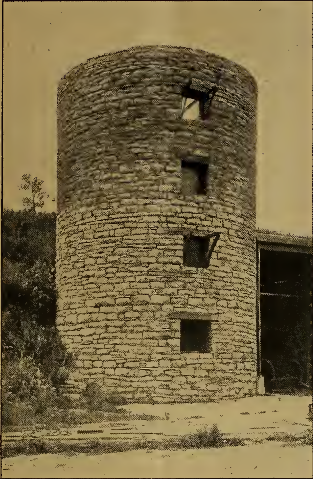
Built in Marion County twenty-three years ago, this silo is the oldest in Missouri. It cost $600 without a roof. Not a cent has been expended for repairs
