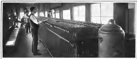
The Pneumatic Switchboard of Today, showing how the Safety of Thousands of Trains is controlled by one Man
