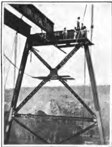
A view of the Gokteik Gorge and the American-built bridge, which opens a new route from India to China
