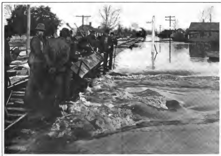
Repairing a Washout on the Railroad at Marion, Arkansas. The Force of the Flood Current against the Track is well shown in the Photograph
