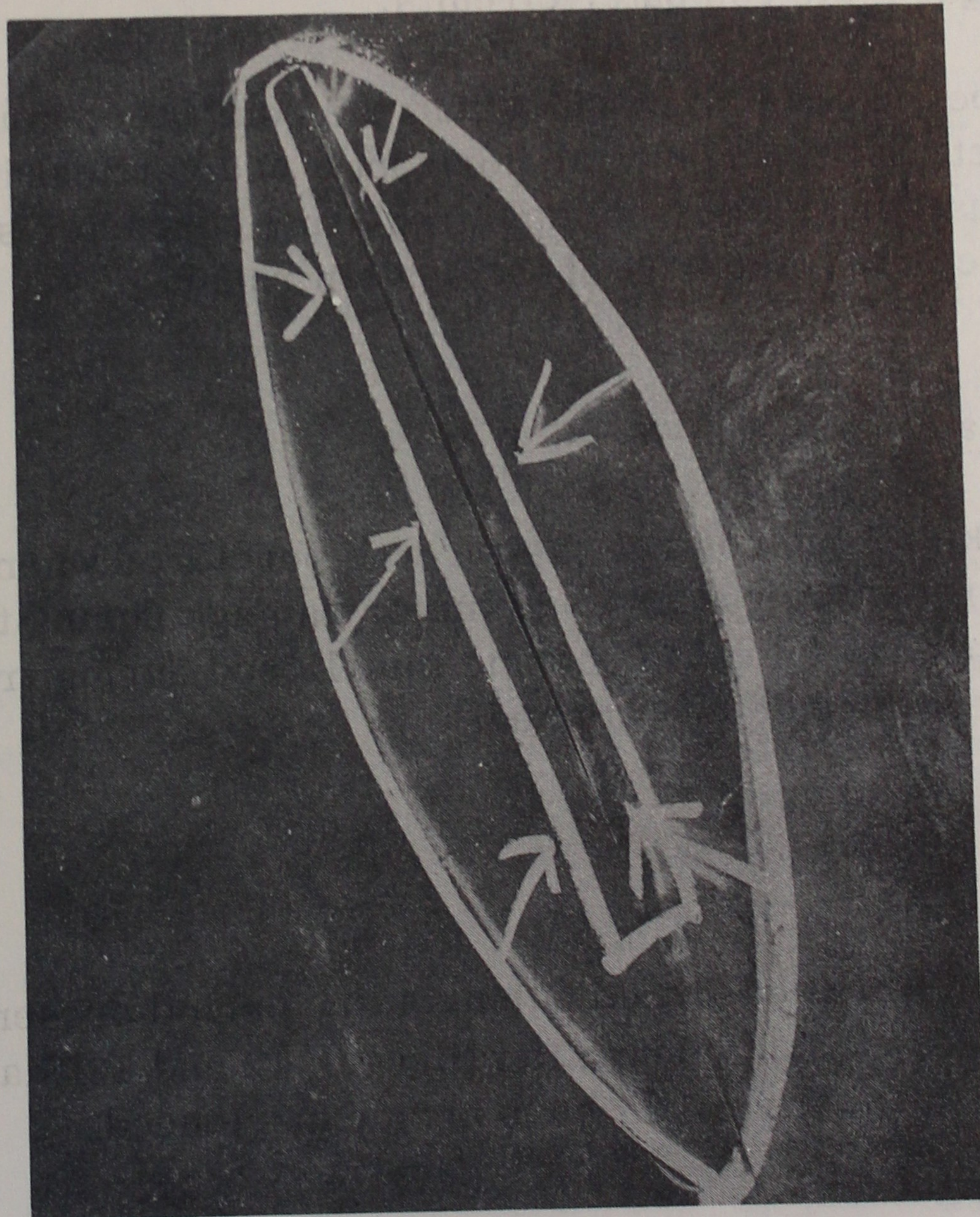
Figure 13. Close-Up View of Seam Separation on Control Shelter.
