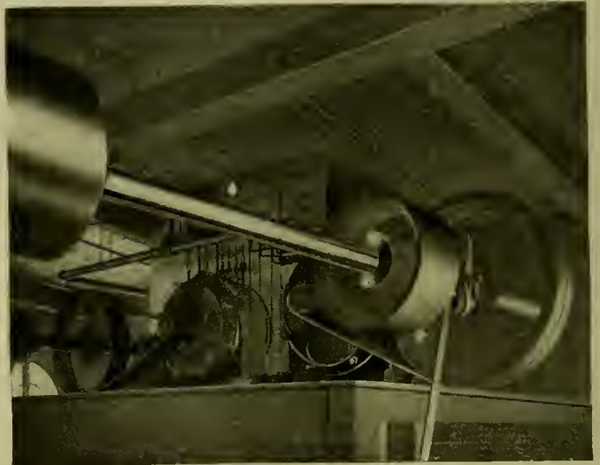
TWO 50 H.P. MAIN SHAFT DRIVES ON 48-IN. CENTERS SHOWN IN MOTION.—TWO CHAINS FROM EACH MOTOR, RUNNING AT 1,445 FT. PER MINUTE.
