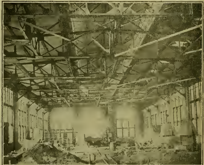
INTERIOR VIEW IN THE BLACKSMITH SHOP, SHOWING PROVISION IN THE ROOF STEEL-WORK FOR THE JIB CRANE SUPPORTS.
