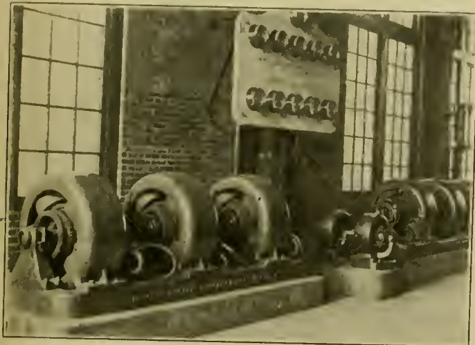
DUPLICATE BALANCERS FOR THE MULTIPLE-VOLTAGE SYSTEM AND SMALL COMPENSATING BALANCER FOR THE ARC LIGHTING SYSTEM.
