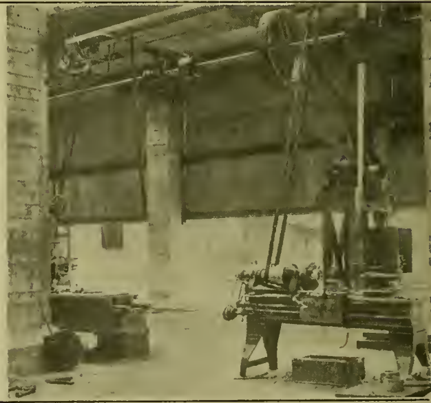
GROUP MOTOR IN MACHINE SHOP.
