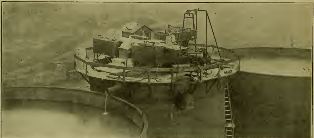
AN INTERESTING VIEW OF THE TOP OF THE MCKEES ROCKS WATER SOFTENER (TAKEN FROM ROOF OF THE ERECTING SHOP), SHOWING ARRANGEMENT OF APPARATUS. LARGE SQUARE SODA TANKS AND HOISTING APPARATUS IN FOREGROUND.
