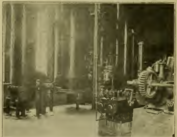
FEED WATER HEATERS AND BOILER-FEED PUMPS IN BOILER ROOM. STOKER ENGINE AT RIGHT.
