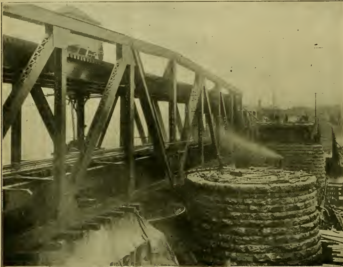
DRAW-BRIDGE OVER THE PASSAIC RIVER, AT NEWARK, N. J.—DELAWARE, LACKAWANNA & WESTERN RAILROAD. VIEW FROM PIER ON NEWARK SIDE AS DRAW SPAN WAS BEING LOWERED ONTO THE NEW PIVOT PIER. OLD PIVOT PIER AT RIGHT; SAND JACKS COVERED WITH CANVAS.
