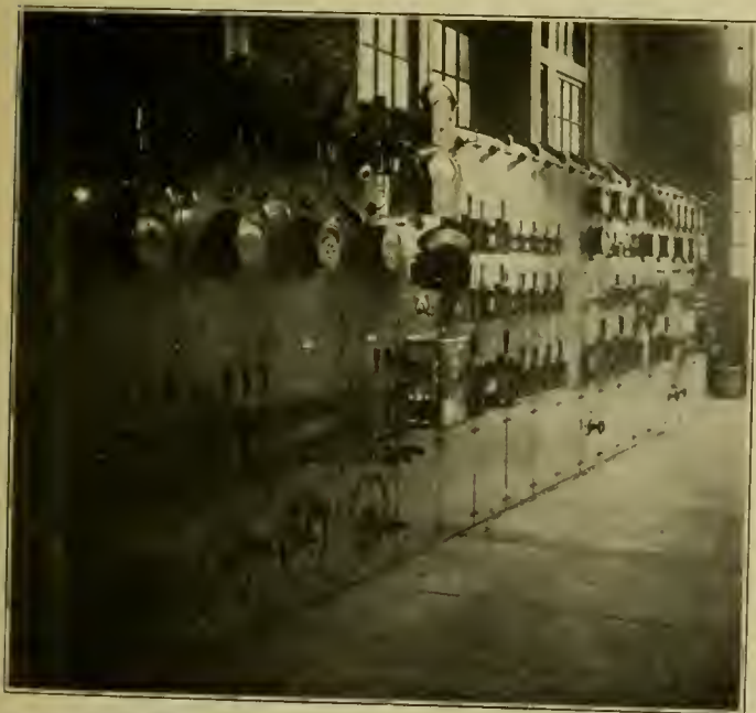
THE SWITCHBOARD, CONTROLLING ALL POWER AND LIGHTING DISTRIBUTION CIRCUITS.
