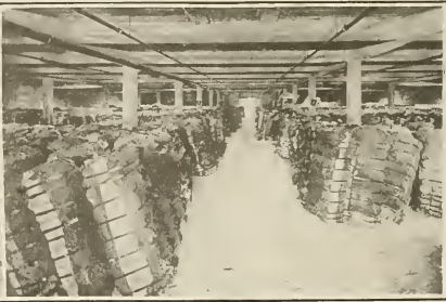
INTERIOR OF A HOUSTON, TEXAS, COTTON WAREHOUSE, PROTECTED AGAINST FIRE BY AUTOMATIC SPRINKLERS.
