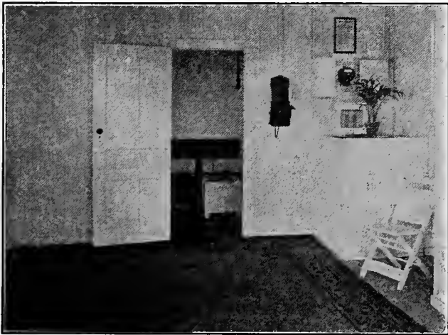
INTERIOR OF SCREENING AND DISINFECTING PLANT. Trap doors at the left of rug. Bleach is stored in the cabinet under the potted plant. Mixing and dosing are done in the rear room, where the dosing device can be seen.
