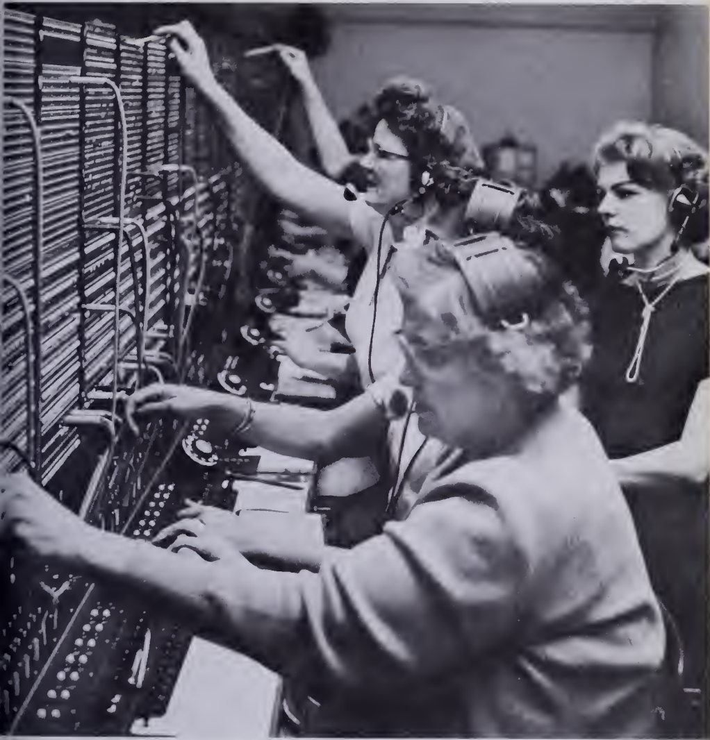
at the telephone switchboards —
