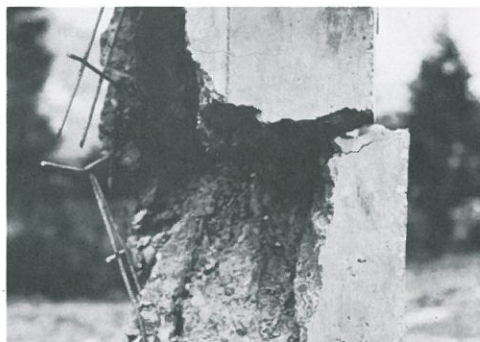
SINGLE ROUND DAMAGE TO 12" THICK REINFORCED CONCRETE
