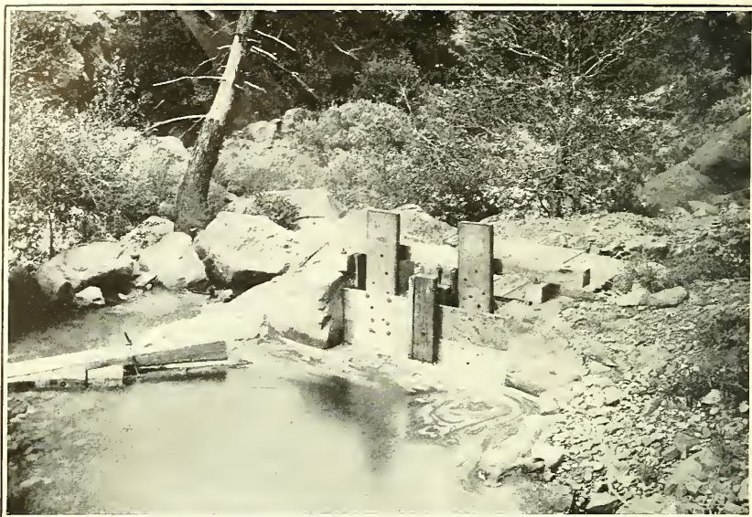
FIG. 1.—HEADWORKS, SOUTH BOULDER AND COAL CREEK DITCH, COLORADO.
