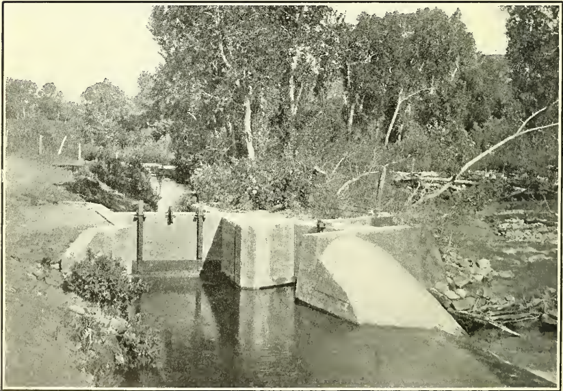
FIG. 2.—DIVERSION WEIR, SAND GATE, AND HEADGATE OF THE JACKSON DITCH NEAR FORT COLLINS, COLO.
