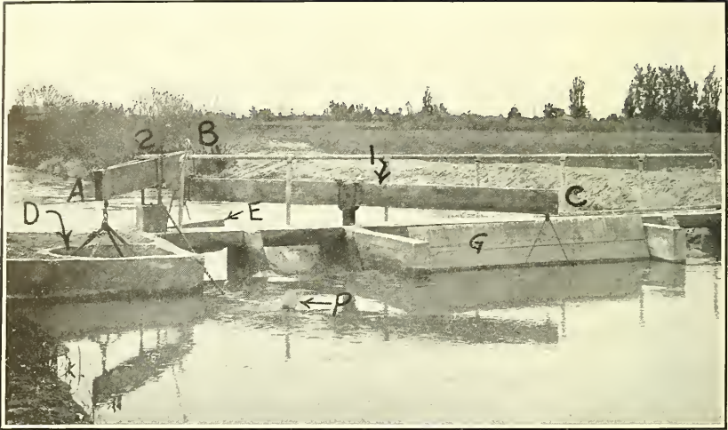
FIG. 1.—AUTOMATIC CHECK GATE, TURLOCK IRRIGATION DISTRICT, CALIFORNIA.
