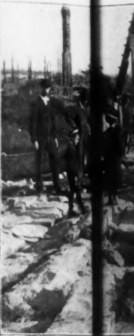
FIG. 5.—SETTING OF CENTER LINE (Showing the extrados of the arch with the center line)
