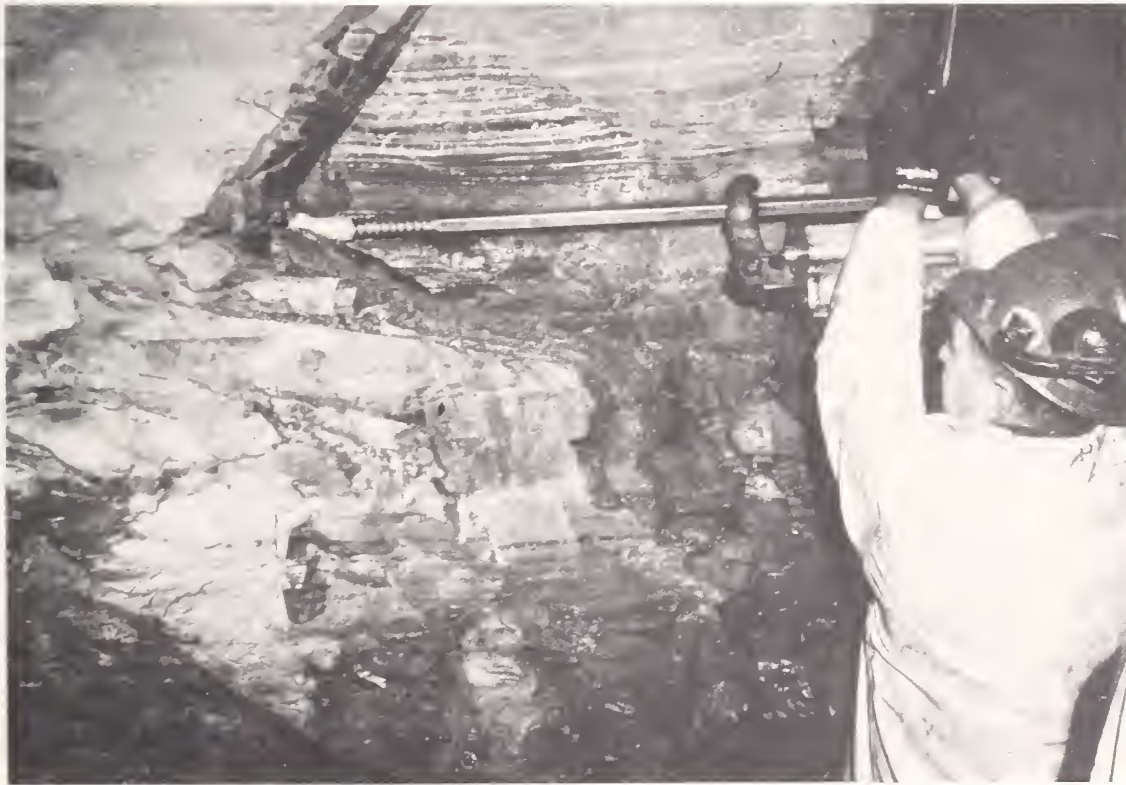
A new technique to control fractures when blasting tunnels is being demonstrated in the MBTA [Boston, Mass.] Red Line extension. Instead of the conventional method of smooth wall blasting, a broaching tool is used to scribe notches in the sides of the drill holes which act as starting points for crack initiation.
