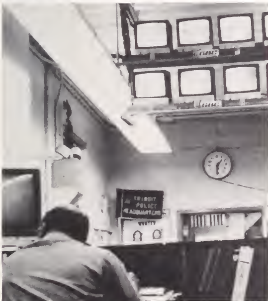
To increase passenger safety and security, closed-circuit television and voice alarms are being tested on a New York City subway line. Note the camera mounted near the station ceiling [top]. The control room in the transit police headquarters where the video and audio signals are received is shown at bottom.
