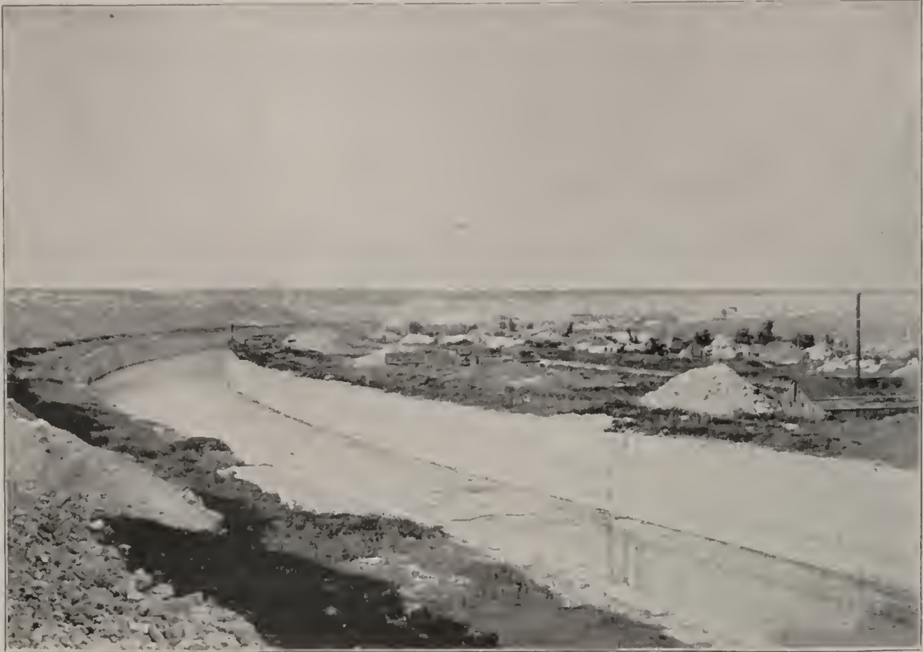
Fig. 71. Great Bend at Romeo, Ill., Chicago Main Drainage Canal, Showing Rock Walls Channeled with the Sullivan Channelers.
