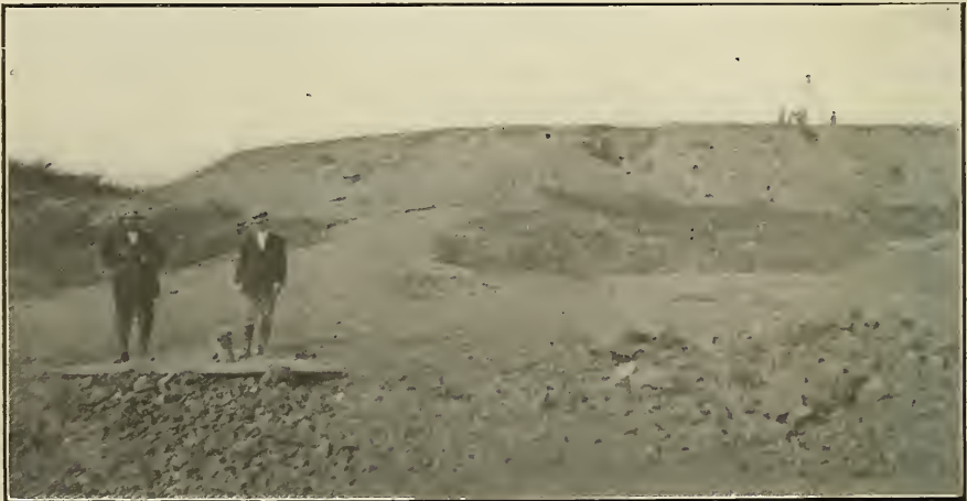
Water supply of Cienfuegos. View of the reservoir. The inlet pipes from the Hanabanilla River has been laid to the tank, and the outlet pipe to the city's streets is likewise in place.
