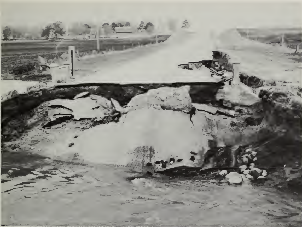
ROAD AND BRIDGE DAMAGE FROM SPRING SNOWMELT 1969. THIS TYPE OF DAMAGE OCCURRED THROUGHOUT THE BASIN AND REPRESENTS A LARGE ECONOMIC LOSS.
