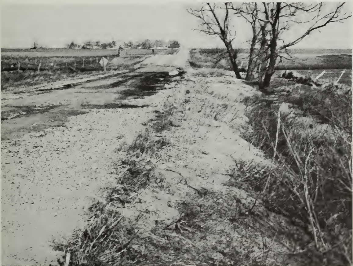
GRAVEL WASHED OFF ROAD AND DEBRIS IN FENCE LINES ARE TYPICAL DAMAGES FROM FLOODWATER.
