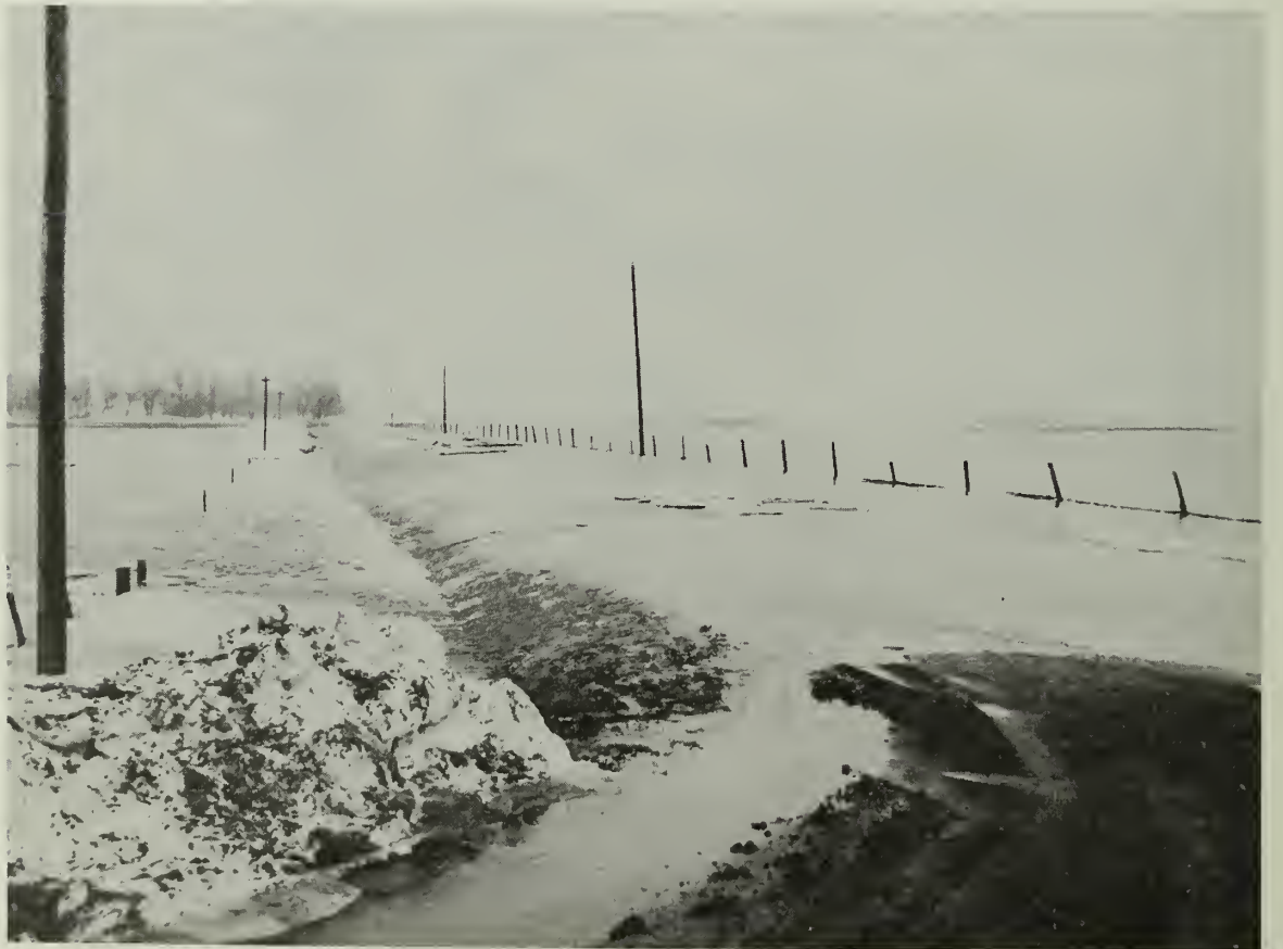
RUNOFF FROM SNOWMELT IN 1969 OVERTOPPED THIS ROAD NEAR BROOKINGS, SOUTH DAKOTA, CAUSING EXTENSIVE DAMAGE.
