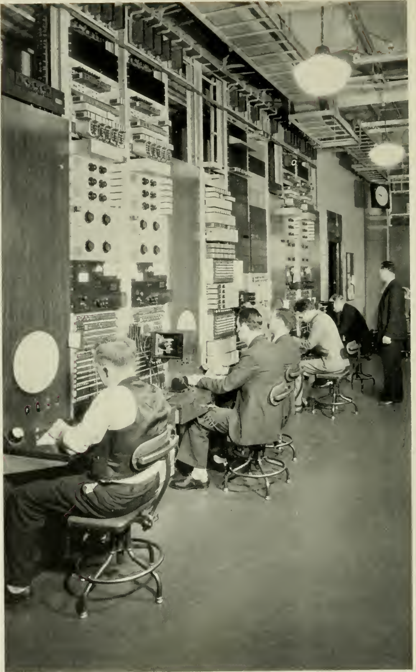
A SECTION OF THE TELEPHONE COMPANY'S MAIN SWITCHING OFFICE IN CHICAGO. Here, in the course of a week, as many as 600 switching operations take place in routing radio programs, as explained in the article which begins on the opposite page.
