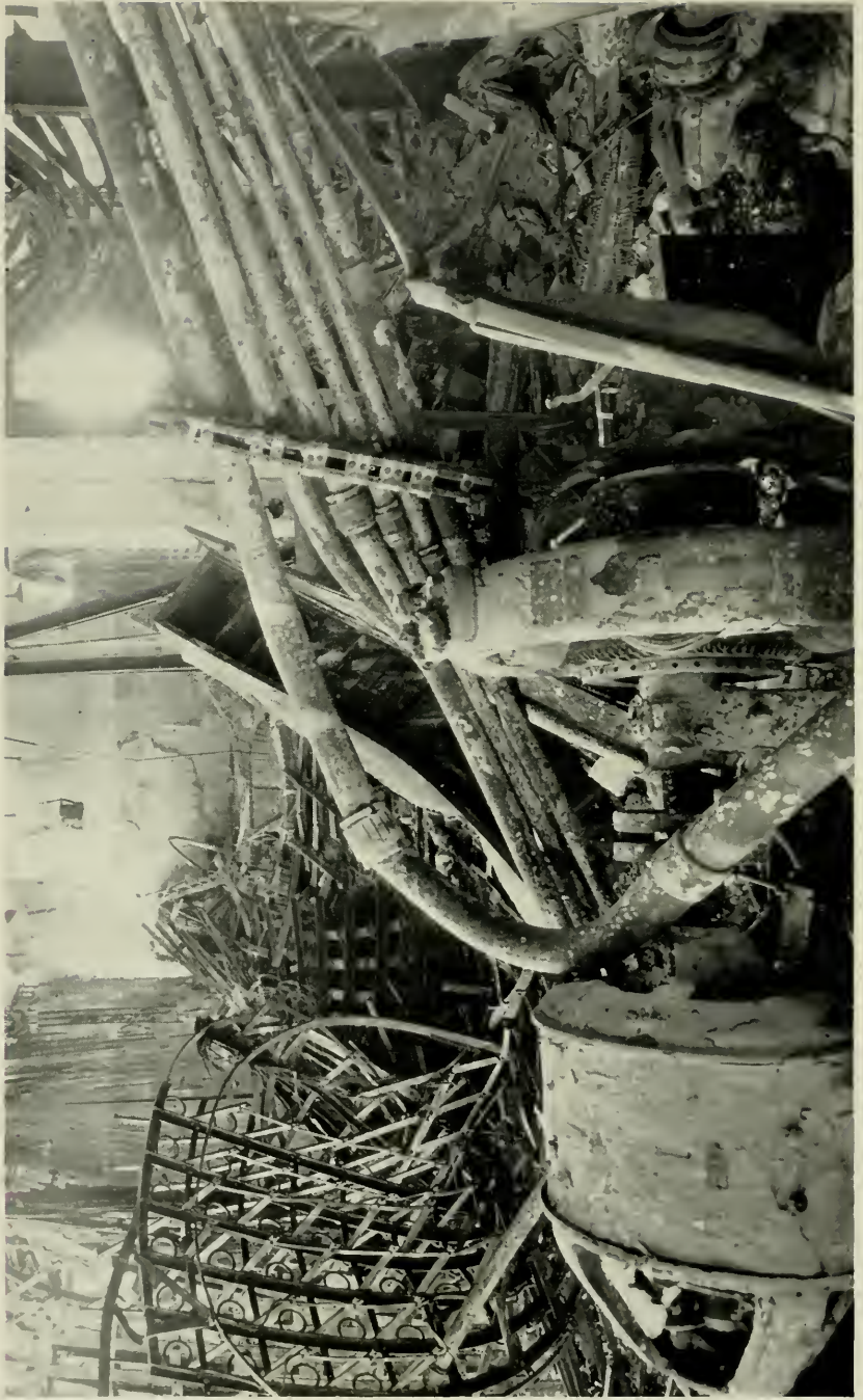
FIGURE 4. THE TERMINAL ROOM OF THE ANDERSON, IND., EXCHANGE AFTER THE FIRE.
