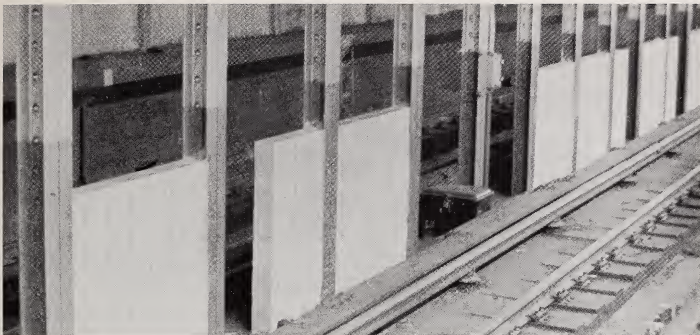
Older stations can be acoustically upgraded with installation of noise control treatments such as sound-absorbing barriers, resilient rail fasteners, and welded rail.
