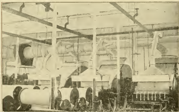
A slasher room, showing the rear of three slashers, with slasher ventilating fan and piping overhead.
