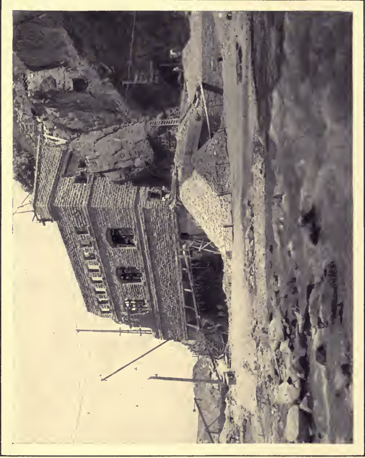
Power-house at Dam Site, Salt River Project, Arizona.
