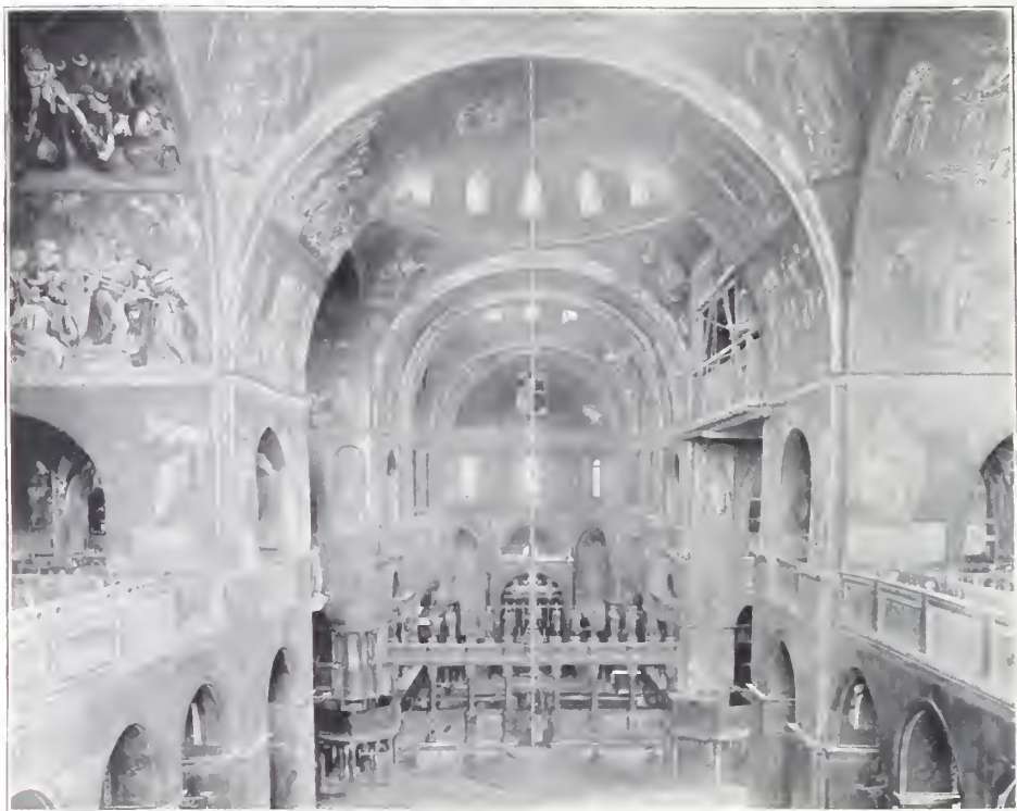
FIG. 1. NAVE OF S. MARK'S, AT VENICE; FROM THE FACADE GALLERY. Showing an outward spread of about three feet in the upper portion of the piers. Compare the outline tracing, Fig. 2.
