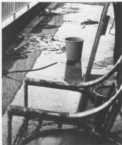
The balcony of William Buckley's apartment, before he was kidnapped. Shelling on the night of February 6 blew out the windows and tore the door off its hinges. Trapped in the embassy by the shelling, Mr. Buckley didn't get home that night.
