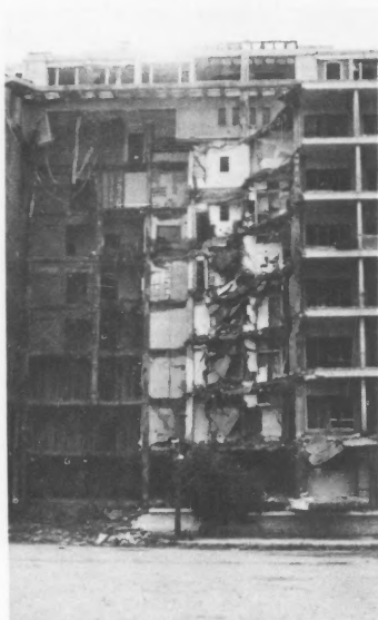
The old embassy building, showing where the kamikaze terrorist struck with his vehicle.
