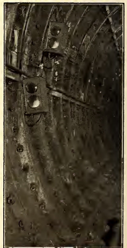
SIGNAL LANTERN IN TUNNEL
