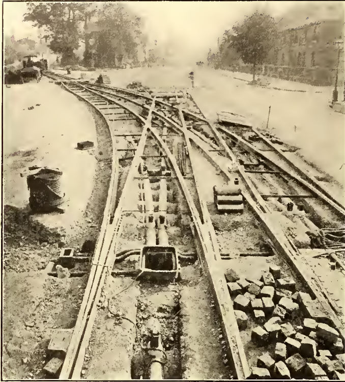
A JUNCTION ON THE LINCOLN CONDUIT SYSTEM
