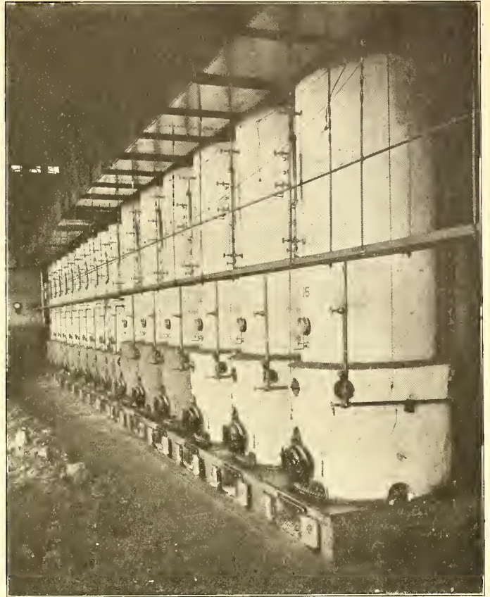
FIG. 3.—THE BOILER ROOM
