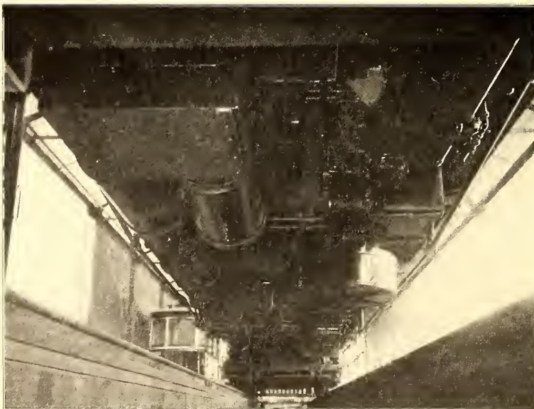
VIEW UNDER UTICA & MOHAWK EXPRESS CAR, SHOWING MULTIPLE-UNIT CONTROL AND STRAIGHT AND AUTOMATIC AIR-BRAKE APPARATUS
