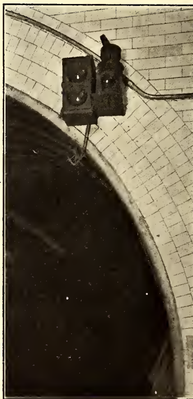
SIGNAL LANTERN AT STATION
