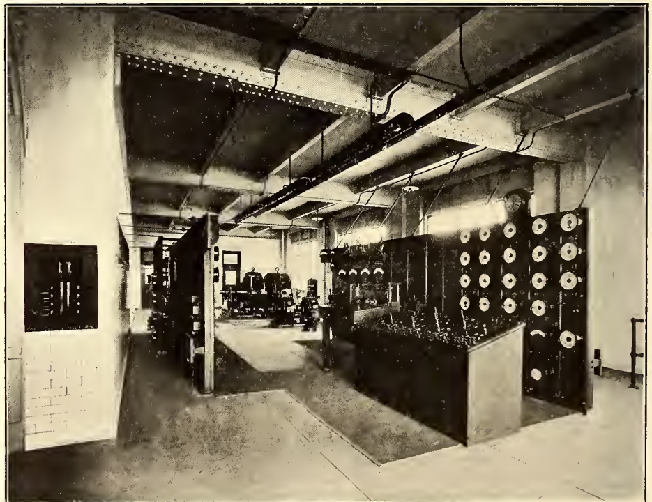
FIG. 22.—ELECTRICAL OPERATING GALLERY
