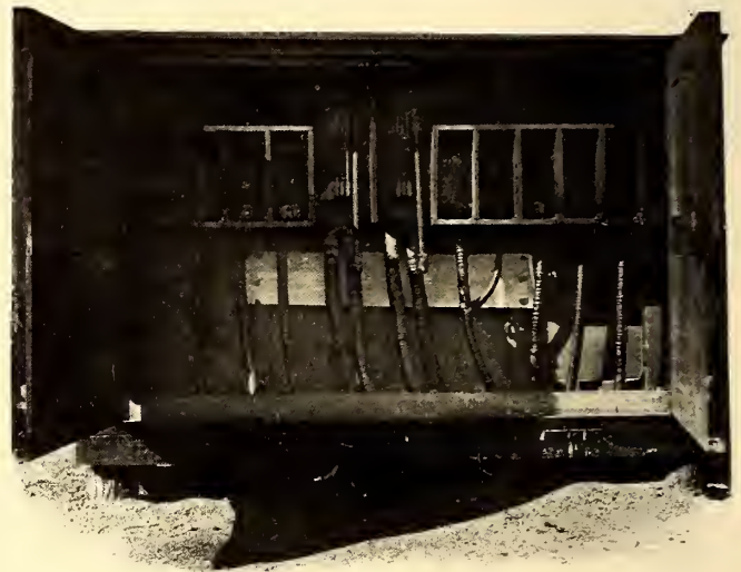
FIG. 35.—SWITCH AND FUSE HOUSE, CONTROLLING THIRD-RAIL SECTIONS IN YARD EAST OF JAMAICA
