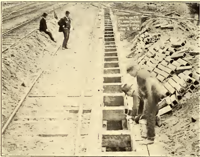
FIG. 4.—CONDUIT MANHOLES CLOSE TO TRACK, ATLANTIC DIVISION
