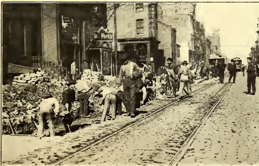
CLEARING AWAY THE DEBRIS AFTER AN EXPLOSION
