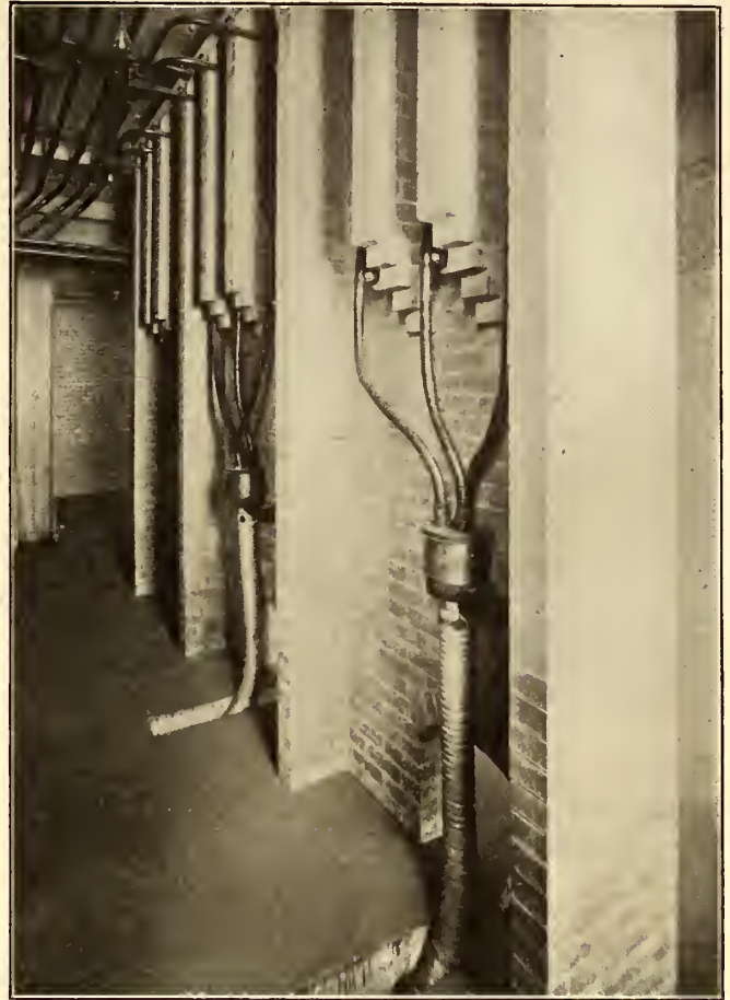
FIG. 20.—HIGH-TENSION FEEDER CABLES IN BASEMENT, ENTERING CONDUITS
