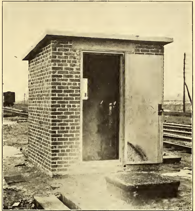
FIG. 3.—VIEW OF PUMP HOUSE ON MAIN CONDUIT LINE, NEAR LONG ISLAND CITY
