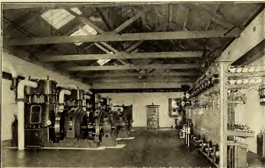
ENGINE ROOM IN POWER HOUSE OF THE FREMANTLE MUNICIPAL TRAMWAYS
