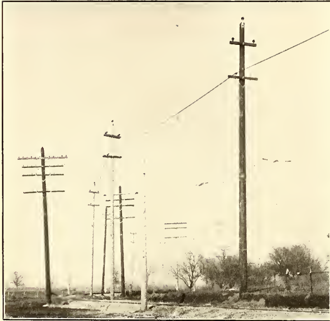
CROSSING OF TELEPHONE LINE WITH TROLLEY WIRES BELOW AND HIGH-TENSION WIRES ABOVE
