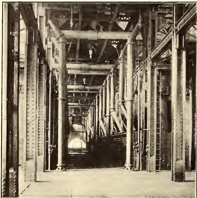
FIG. 6.—BOILER ROOM, SECOND FLOOR
