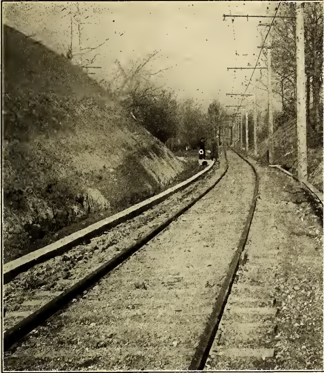
CUT ON SULLIVAN LINE, SHOWING CONCRETE WORK TO PROTECT GRADES FROM WASHING
