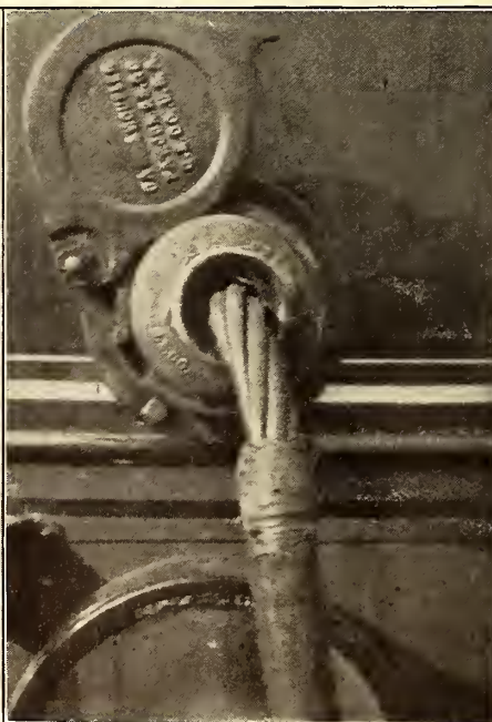
FIG. 4.—JUMPER TERMINAL WITH WIRE EXPOSED
