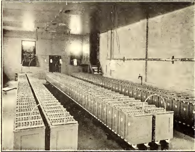
BATTERY ROOM OF THE FREMANTLE TRAMWAYS SYSTEM
