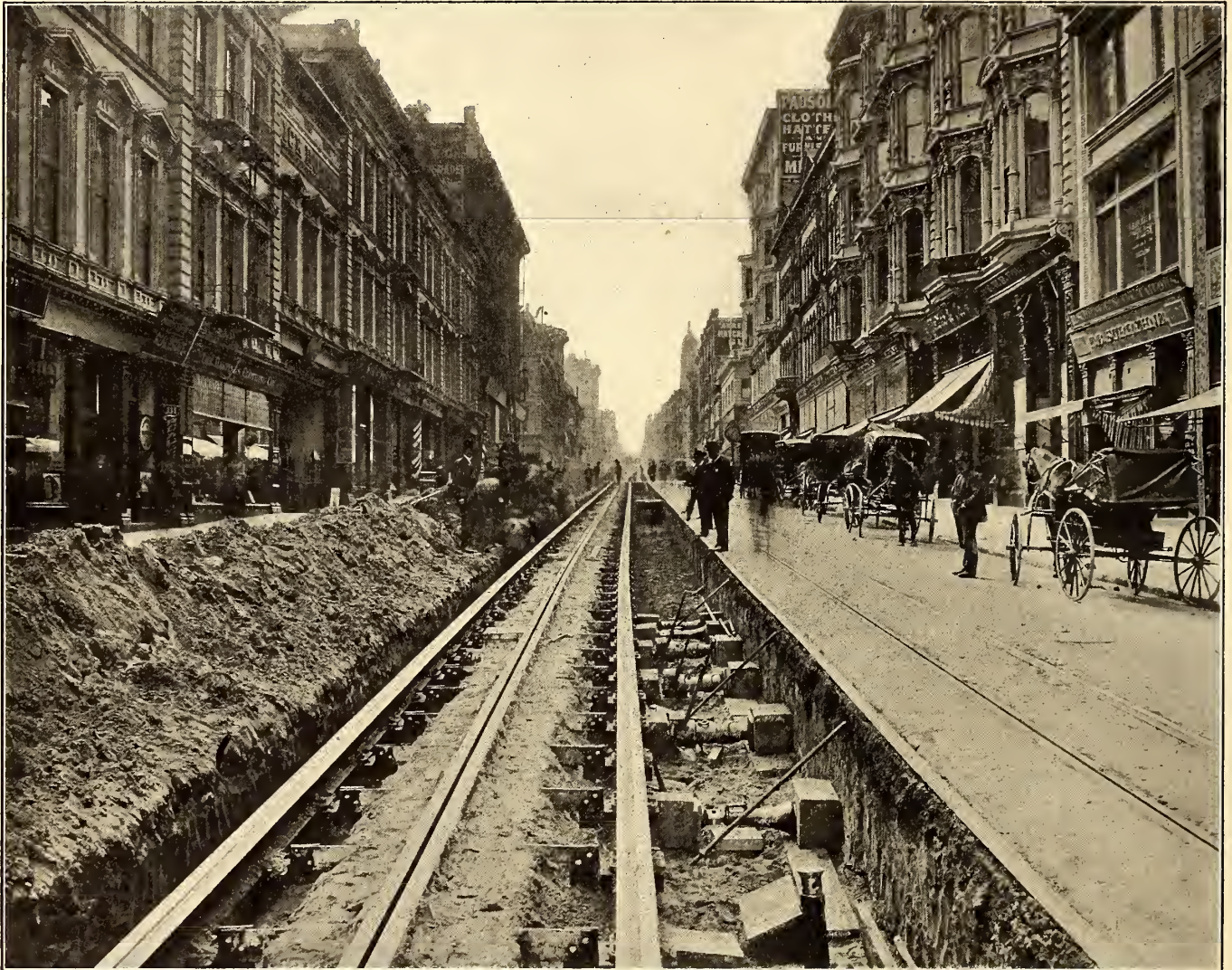
TRACK WORK ON THE SUTTER STREET LINE, SAN FRANCISCO, BEFORE THE FIRE. THE JACKS ARE IN POSITION FOR MOVING OVER THE BED OF THE TRACK
