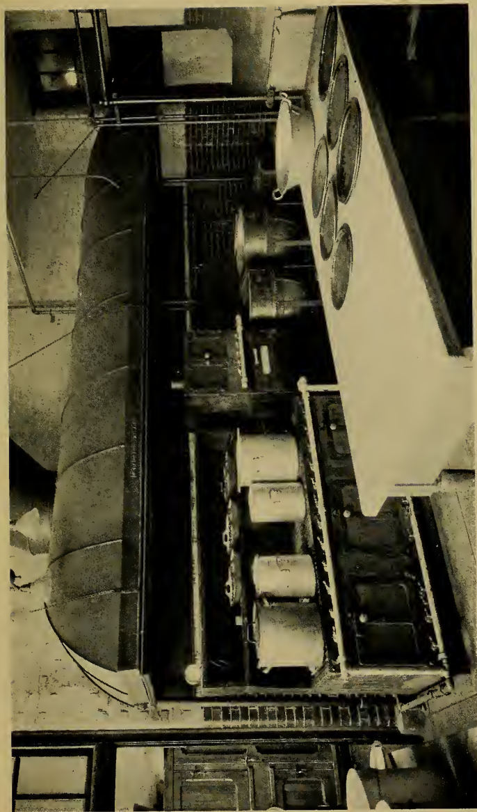
PLATE 3—ONE SIDE OF HIGH SCHOOL KITCHEN, SHOWING VENTILATING HOOD OVER STOVE AND STEAM COOKERS.
