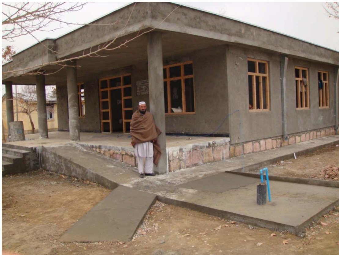
The new physiotherapy clinic built by SCA in Balkh district in Balkh province
