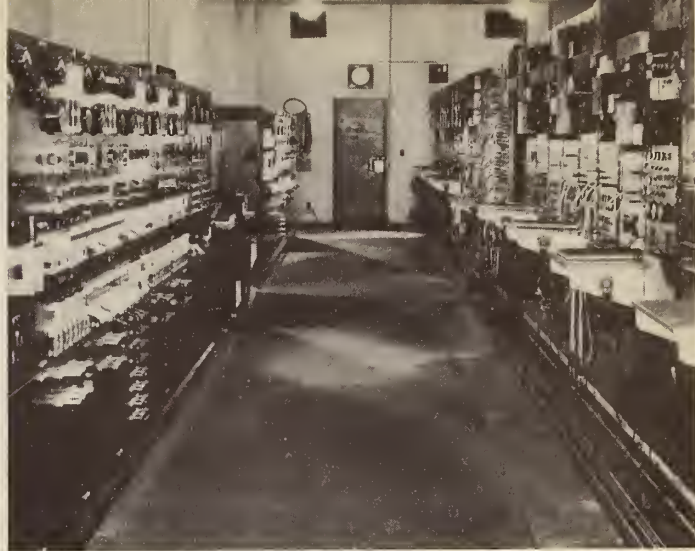
Main amplifier room and control panel for sound recording.
