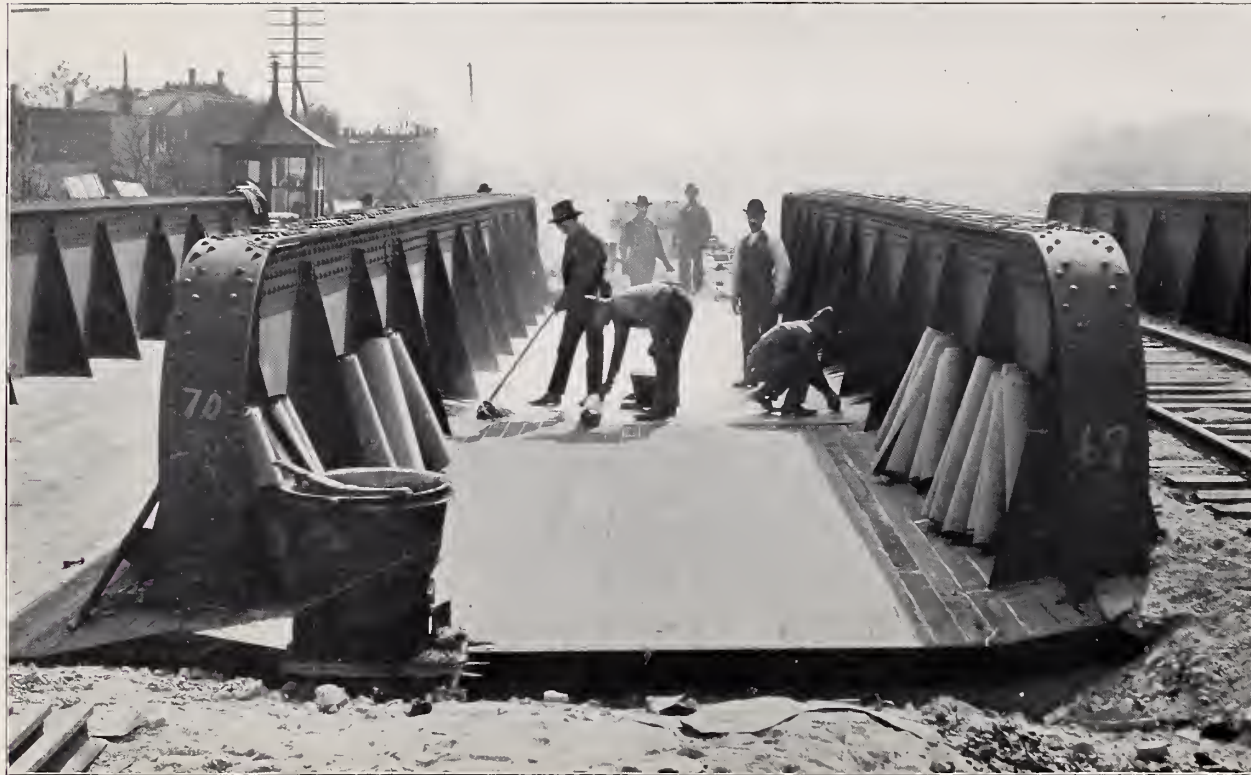
WATERPROOFING SOLID, BALLASTED FLOOR BRIDGES: TRACK ELEVATION WORK, CHICAGO & WESTERN INDIANA R. R. AT CHICAGO. "HYDREX" WATERPROOFING MATERIALS OVER DECK
