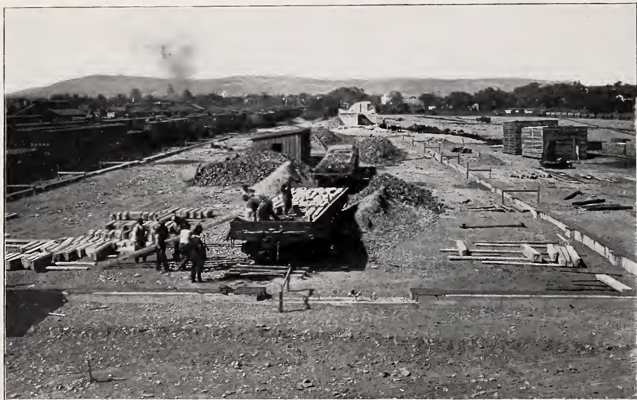
STARTING HYDREX WATERPROOFING FELT AS A DAMP COURSE THROUGH THE WALLS IN ONE OF THE SHOPS OF THE LEHIGH VALLEY R. R., SAYRE, PA.
