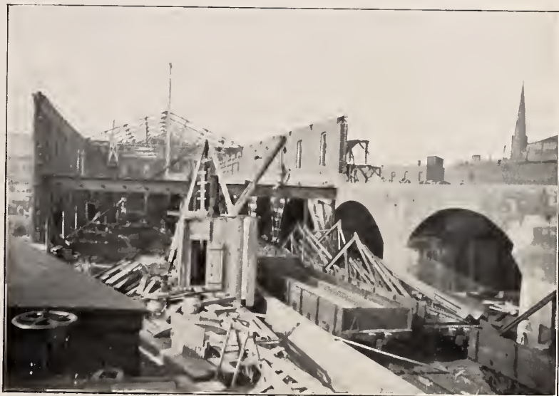
DELAWARE, LACKAWANNA & WESTERN R. R. SHOPS, NEWARK, N. J. HYDREX USED FOR WATERPROOFING AND DAMP COURSING
