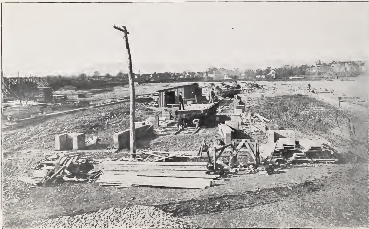
NEW SHOPS, LEHIGH VALLEY R. R., SAYRE, PA., SHOWING VIEW OF STOREHOUSE FOUNDATIONS WATERPROOFED WITH HYDREX
