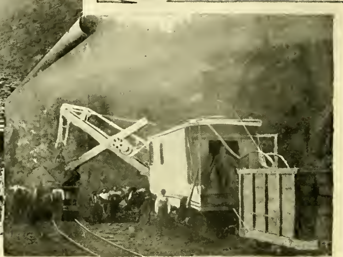
STEAM SHOVEL AT WORK IN OPEN CUT AT ORISKANY, CRAIG COUNTY, VA
