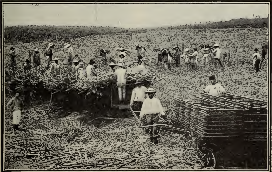
LAYING PORTABLE RAILWAY TRACKS FOR THE CARRYING OF SUGAR CANE TO THE MILLS.
