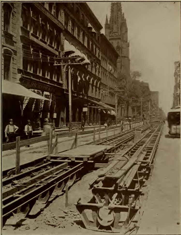
Broadway below Trinity Church. Replacing of the old cable with the underground trolley. (1900.)
