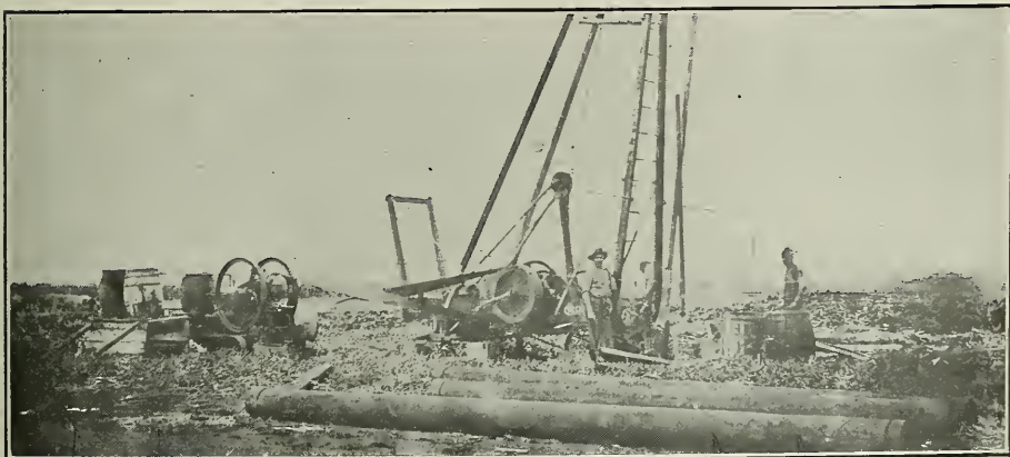
Drilling a 10' Well for Obtaining Irrigation Water, Colonia HORGUITA, Central CONSTANCIA, Cienfuegos.
