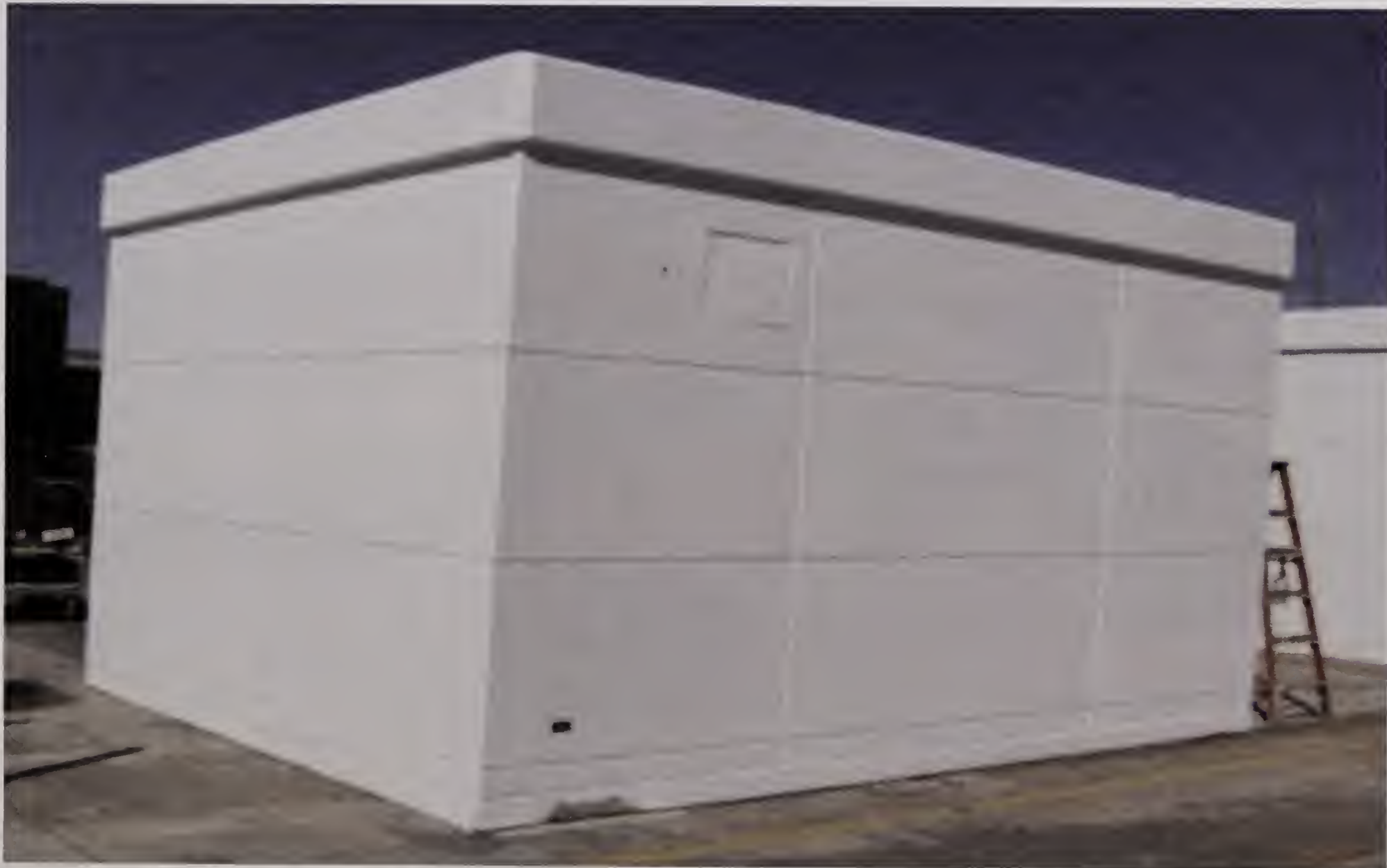
Figure 2-5 Photograph of Typical Power Conversion Station
