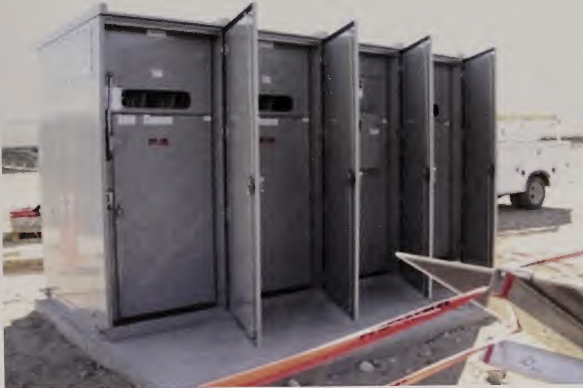
Figure 2-6 Photograph of Typical PV Combining Switchgear
