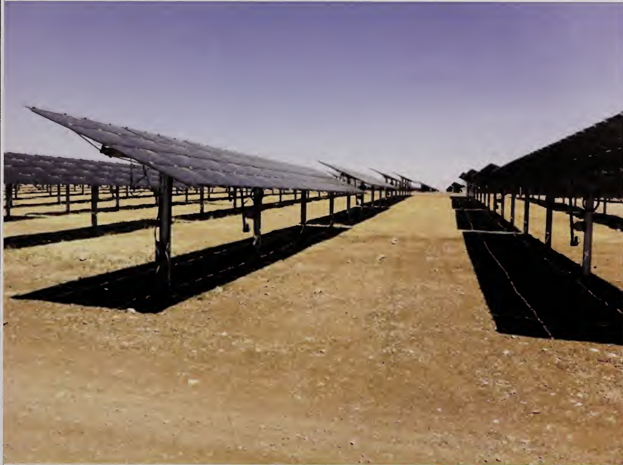
Figure 2-3 Photograph of Typical Solar Array
