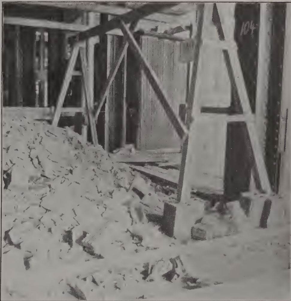
FIG. 30. A DANGEROUS METHOD OF SUPPORTING A HORSE SCAFFOLD.
