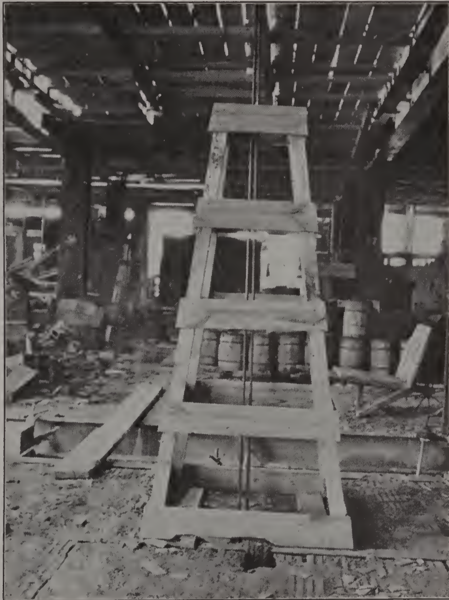
FIG. 13. AN EFFECTIVE GUARD FOR HOISTING CABLES.
