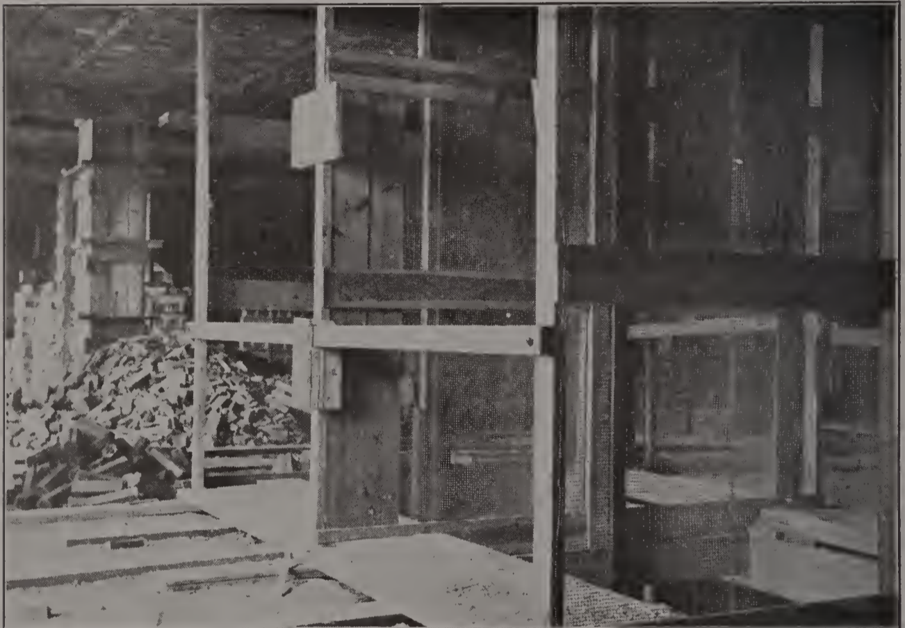
FIG. 16. AN APPROVED TYPE OF MATERIAL-HOIST FENCING.
