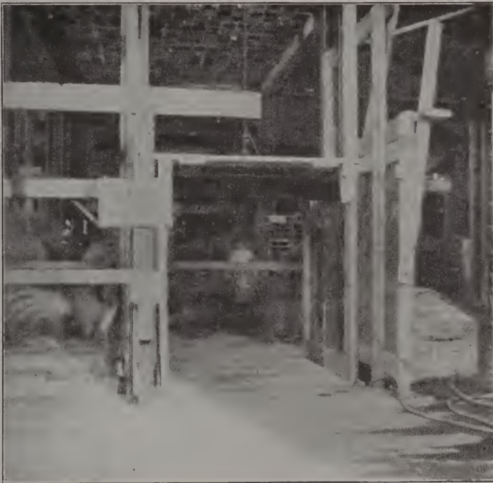
FIG. 17. OVERHEAD COVERING FOR THE CAGE OF A MATERIAL HOIST.
