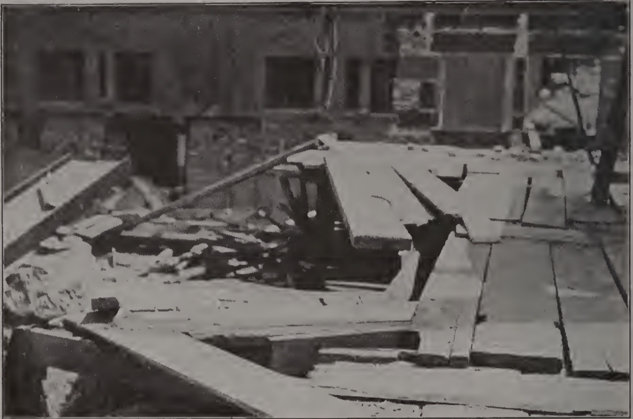
FIG. 34. DANGEROUS CONDITIONS ABOUT A RUNWAY.
