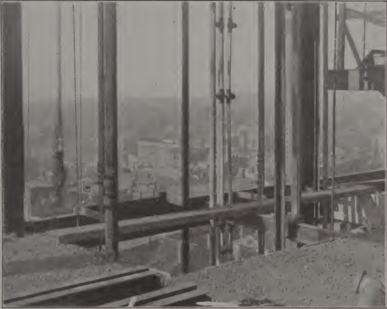
FIG. 40. AN UNGUARDED ELEVATOR SHAFTWAY.
