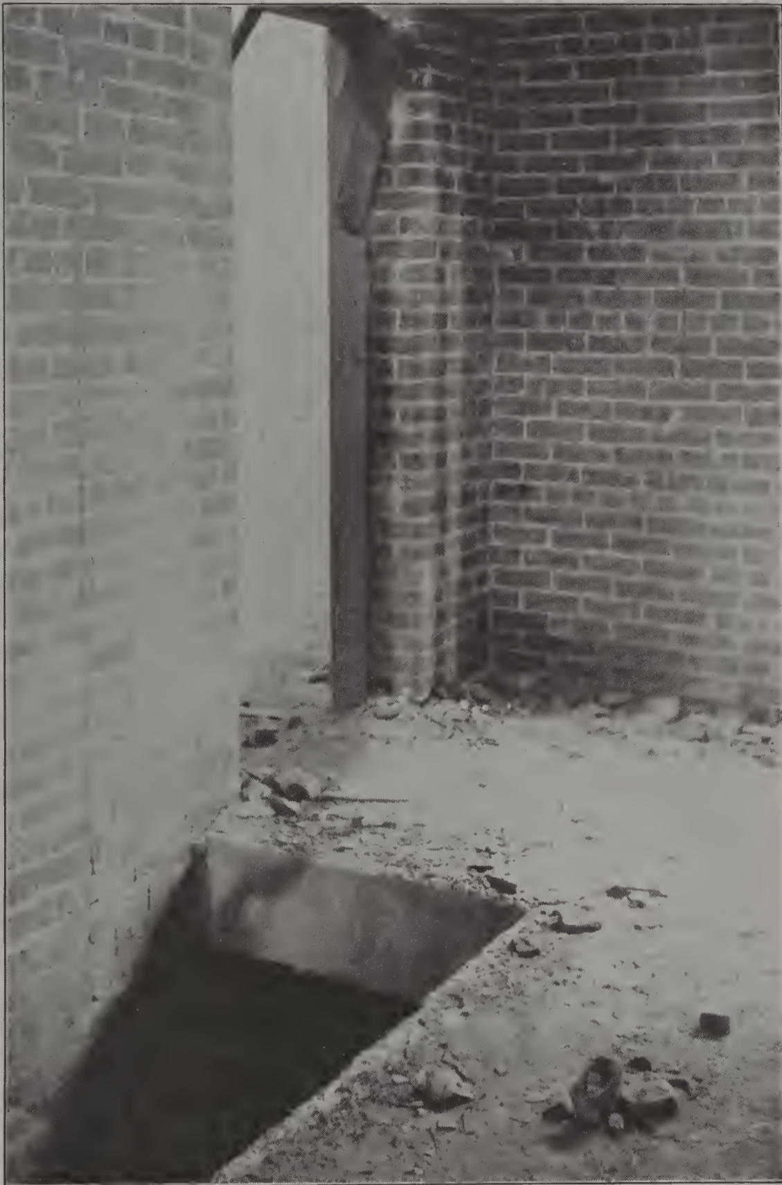
FIG. 38. A DANGEROUS FLOOR-OPENING.
