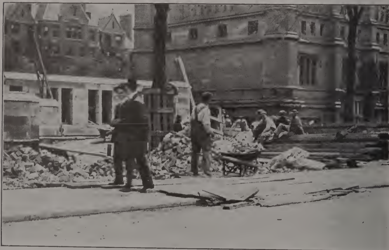
FIG. 7. A POORLY-MADE PROTECTION FOR A SIDEWALK.
