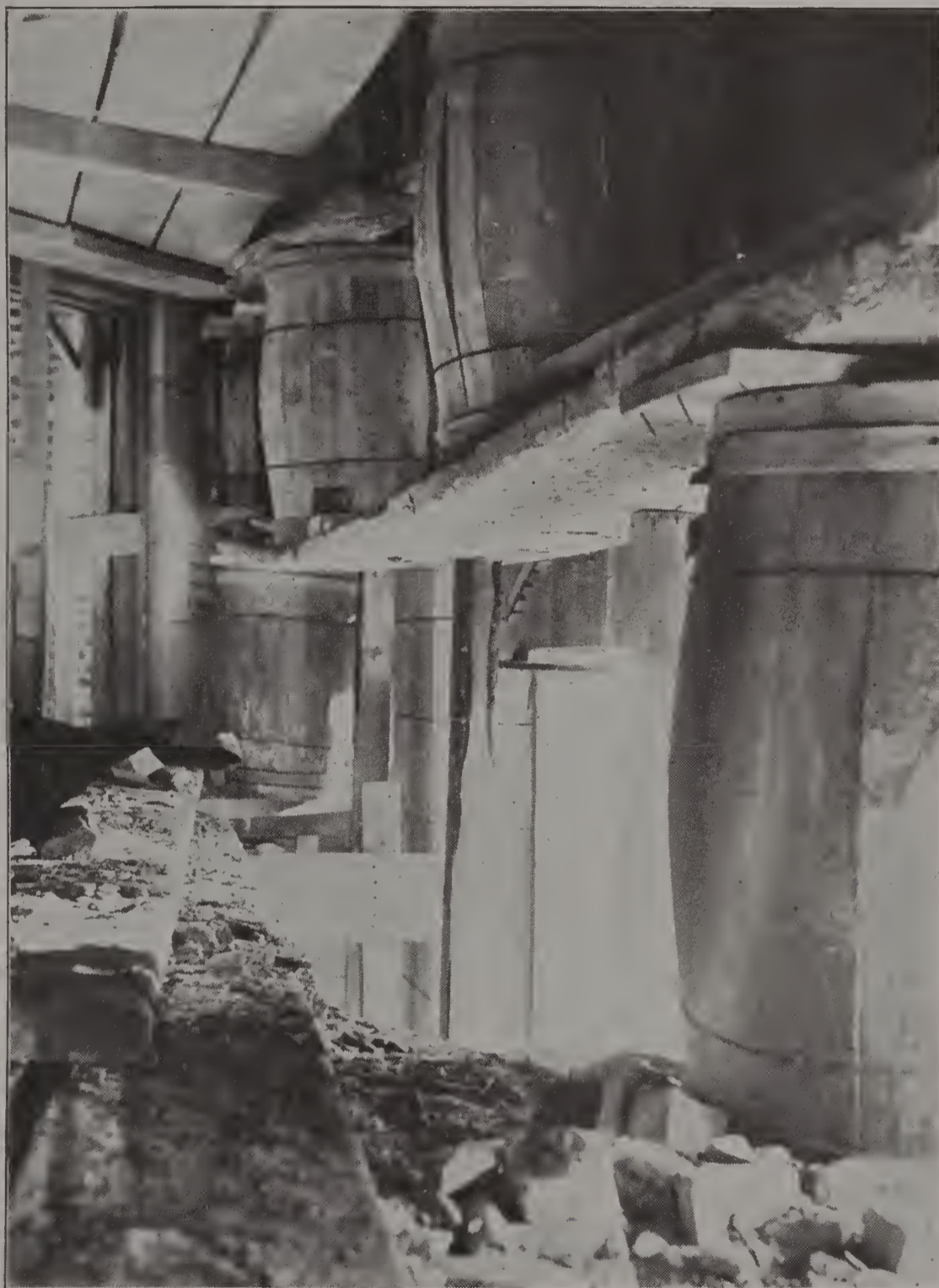
FIG. 31. A STUDY IN DANGEROUS SCAFFOLDING.
