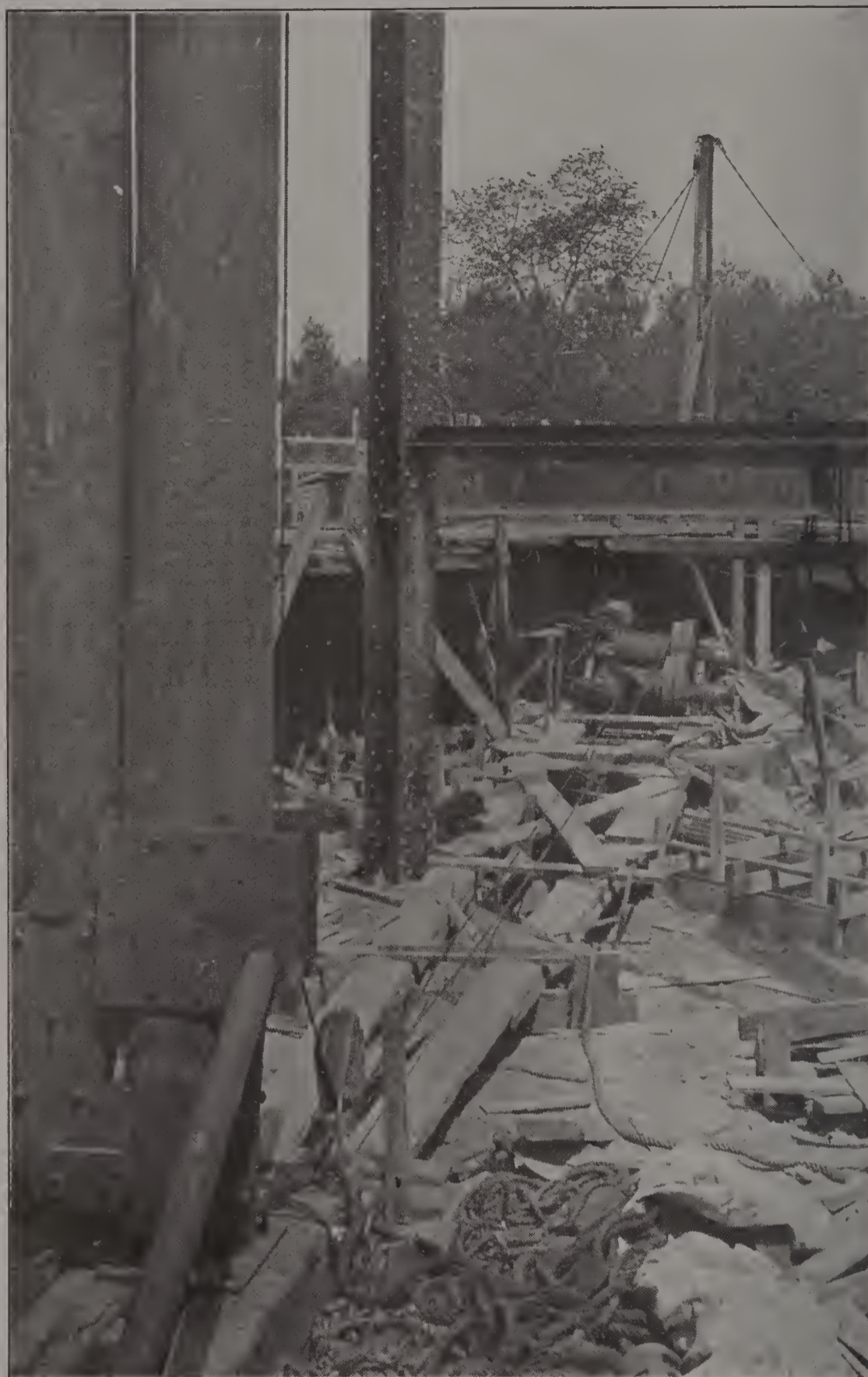
FIG. 9. UNPROTECTED HOISTING ENGINE, CABLES, AND GUIDE BLOCKS.
