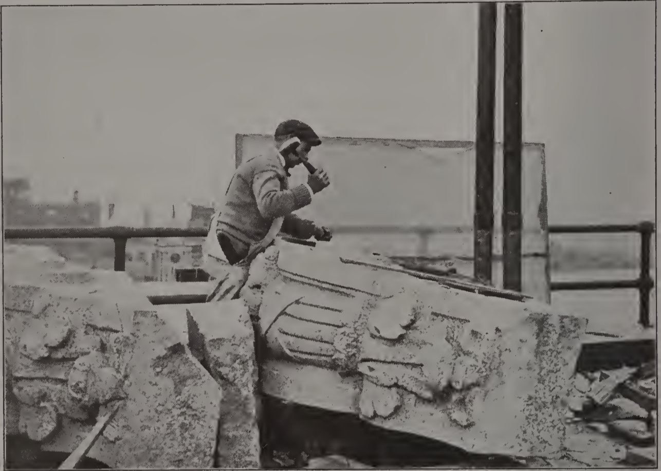
FIG. 49. USING A CLOTH SCREEN TO PREVENT CHIPS OF STONE FROM FLYING INTO THE STREET.
