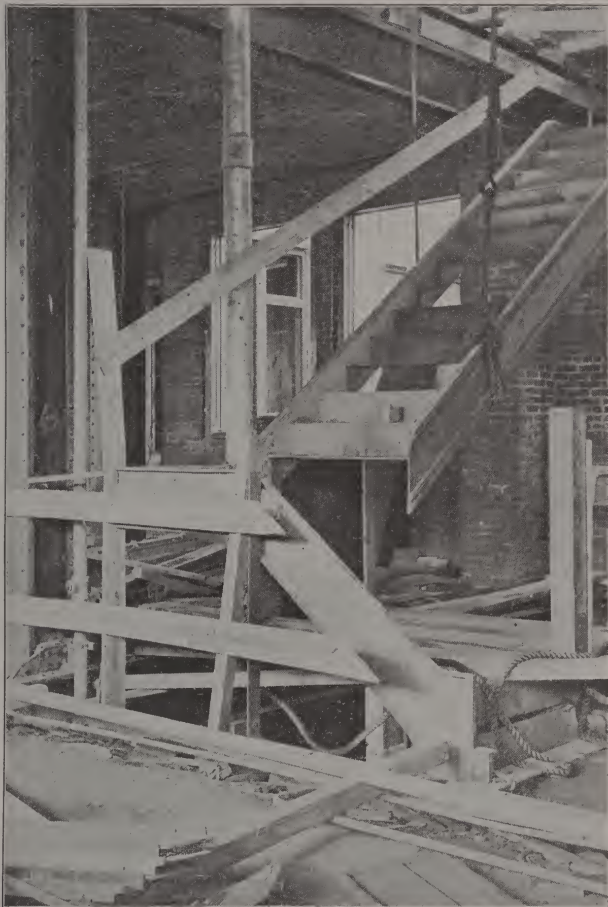
FIG. 19. AN IRON STAIRWAY, BROKEN BY A FALLING LOAD OF MATERIAL.
