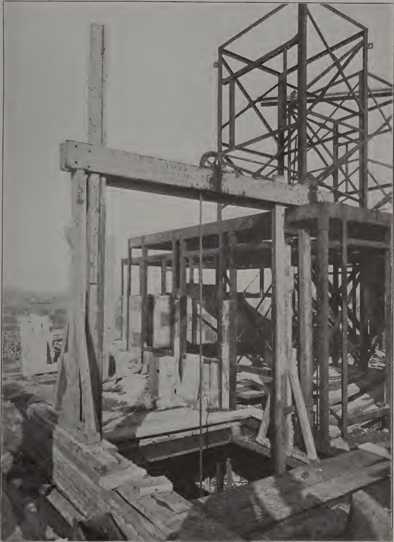
FIG. 14. AN UNGUARDED SHAFTWAY FOR A MATERIAL HOIST.
