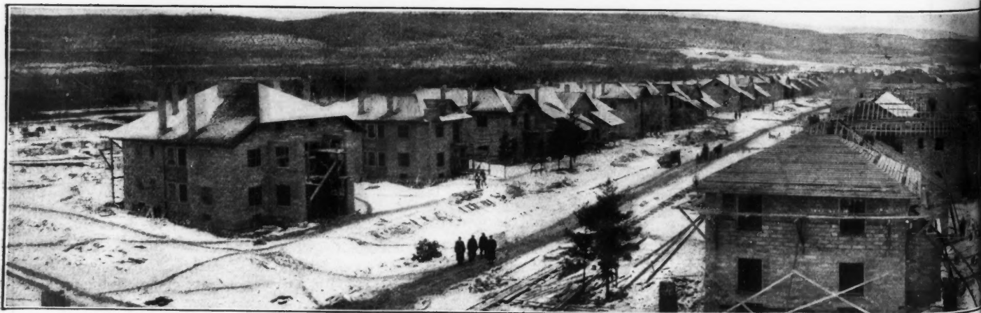
MINNESOTA STEEL CO.'S MODEL TOWN, NEAR DULUTH, MINN., WHERE 170 CONCRETE The town is several miles above Duluth, on Spirit Lake, an embayment of the St. Louis River. It has street-car connections
