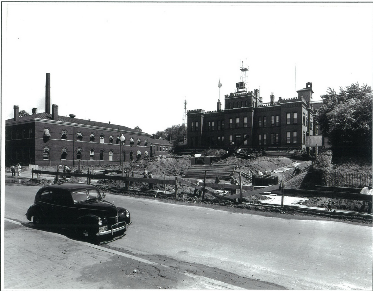
Figure 1. The Ferguson Building with the tower for measuring wind and the Old Annex to the left. The new building construction is in the foreground. Picture taken facing south-southeast.
