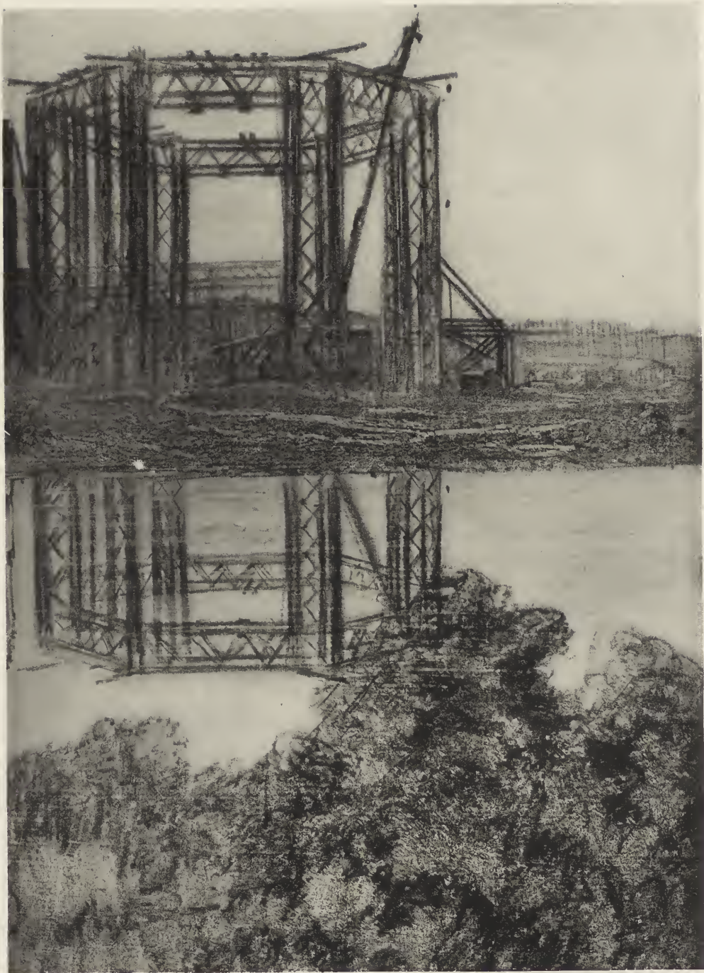
SKETCH OF THE CONSTRUCTION FOR THE CENTRAL DOME OF THE PALACE OF FINE ARTS, APRIL, 1914. DESIGNED BY THE ENGINEERING DEPARTMENT OF THE PANAMA- PACIFIC EXPOSITION. BERNARD MAYBECK, ARCHITECT.
