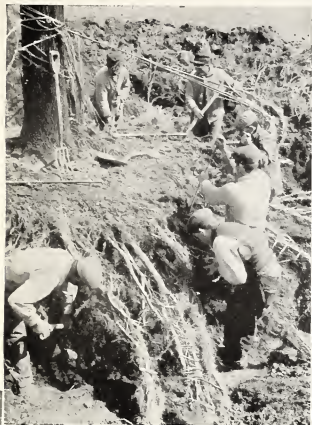
Left—Hicks system of dissecting out and bundling the feeding roots of large Maple. These roots are not cut off with a mattock, but a large crew of men skillfully dissect out and preserves them. For other details of tree moving process developed by Hicks Nurseries, see pages 16-28
