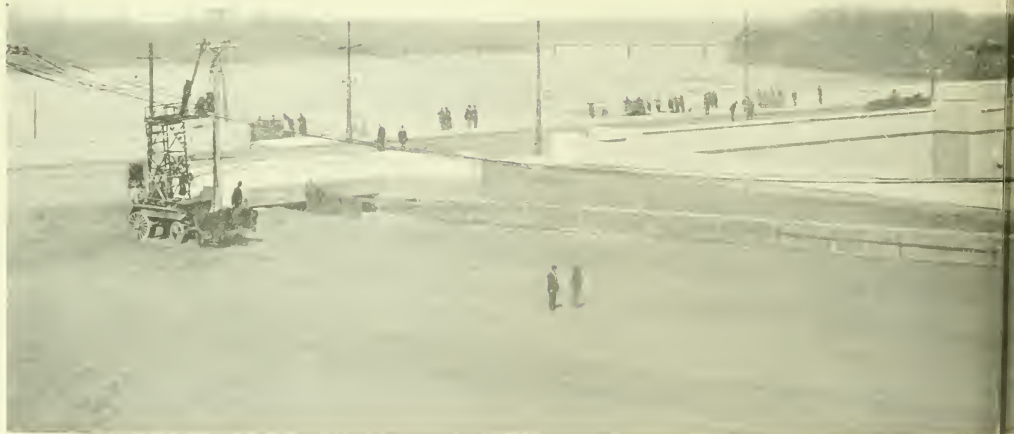
NEW CONNECTICUT This great bridge, built with 2 spans and 8 piers and with a maximum clear height of arch above low water of 55 feet, is the largest stone arch bridge in the world, having a total length of 1,193 feet. The width is 82 feet, including two 10-foot sidewalks and a 60-foot roadway. Total cost of construction about $1,600,000.
