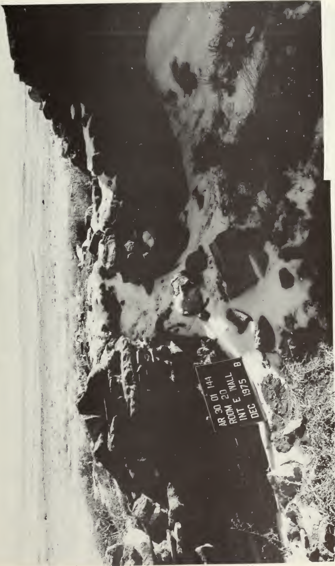
Photo 17 Cave-in of wall Before stabilization Casamero AR-NM-01-144
