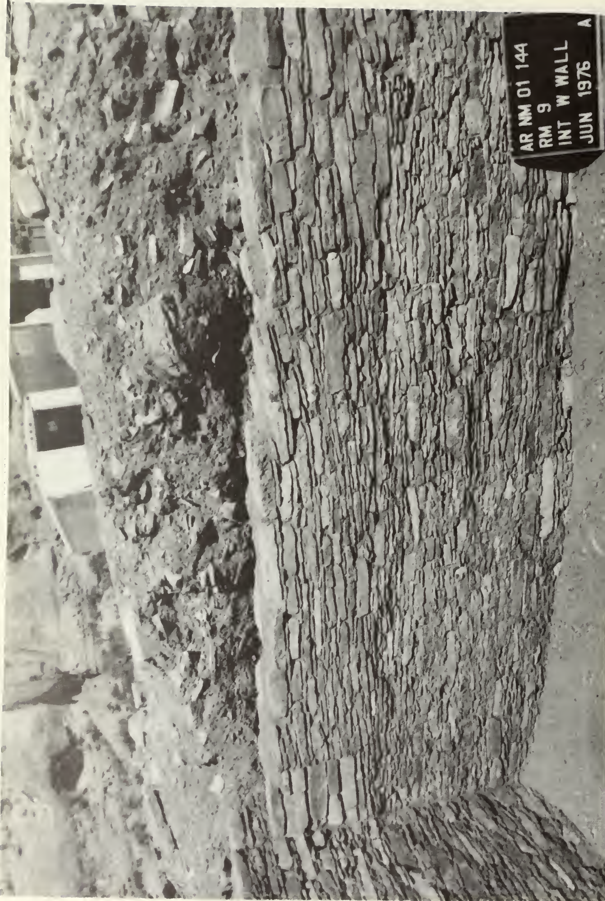
Photo 45 Interior west wall of Room 9 showing a plugged vent discovered during stabilization. This is not shown on the map.
