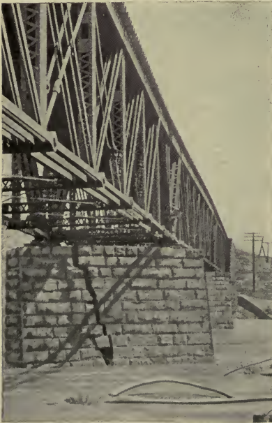
Bridge No. 3, Four and One-quarter Miles West of Columbus. Note Cleavage in Pier
