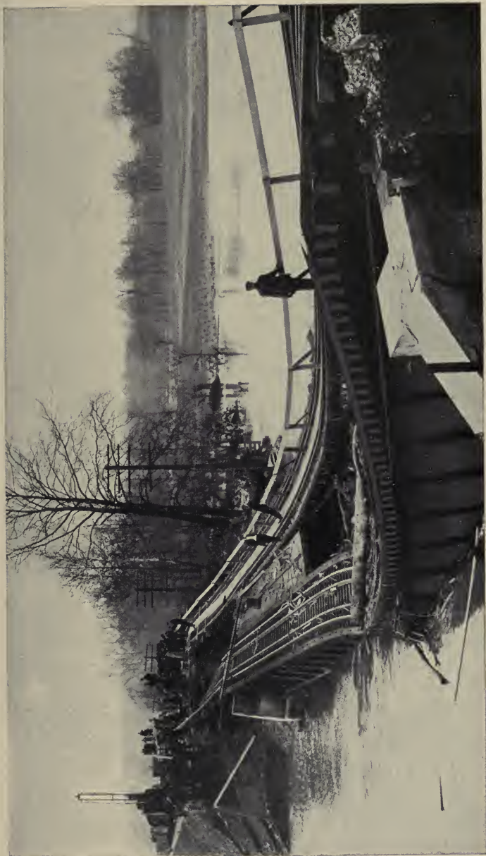
Bridge No. 145, Eastern Division, Over Black Fork Pier and Both Embankments Badly Damaged, 100 Feet of Embankment Washed Out
