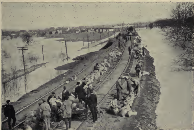
Jeffersonville, Ind.—General View of the Fill. Water on One Side About Twenty Feet Higher Than on the Other Side. If this Bank Had Given Way it Would Have Flooded the Whole Town of Jeffersonville
