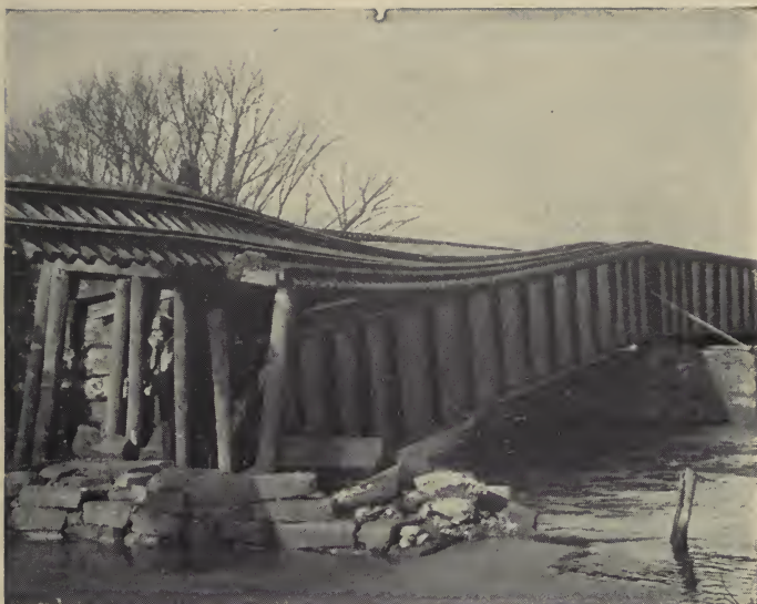
Bridge No. 141, East Division. East Abutment Partly Washed Out. 100 Feet of Embankment Washed Out
