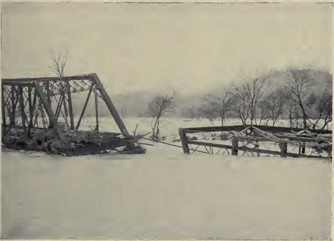
Four and One-half Miles West of Coshocton. Bridge No. 100 Destroyed, Breaking Main Line Between New York and St. Louis
