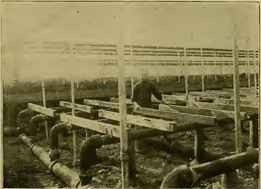
M. WINANDY CO'S NEW BENCH AND HEATING SYSTEM.
