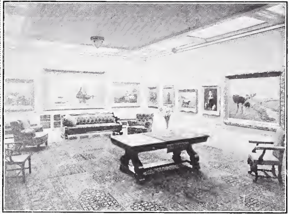
Private Art Gallery, C. H. Frye, Seattle, Wash., showing Frink System for picture lighting installed
