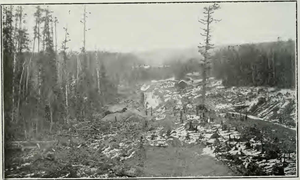
Pipe line excavation, looking north-east towards site of power house, Wawaitin falls, Nov., 1911.
