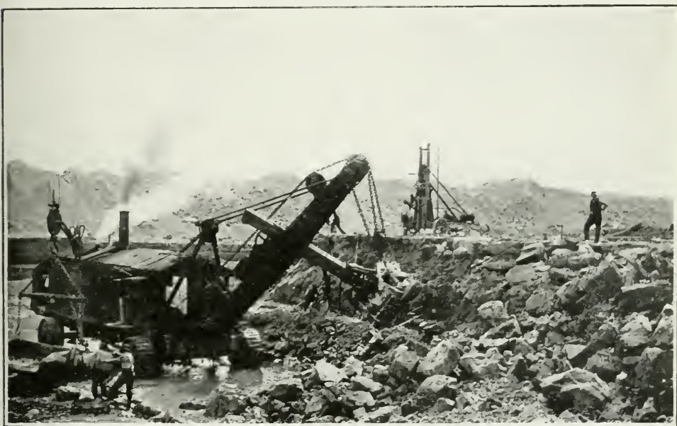
Steam shovel in rockwork, also fast working drill invented for this contract.
