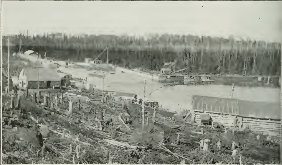
General view of dam, spillway, flume and power house of Porcupine Power Co., Oct., 1911.
