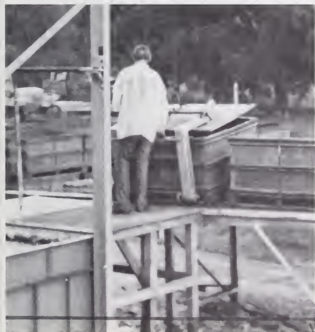
FIGURE 12.—Mobile forklift cage picks up pallet boxes from center of pallet box conveyor.
