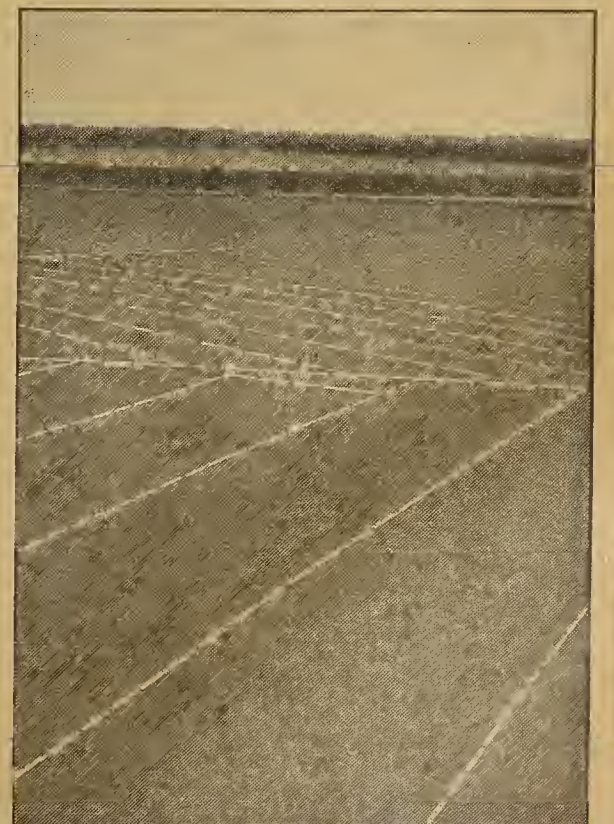
Here is shown a portion of five acres of prepared roofing over an oil reservoir
