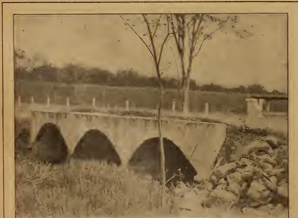
Here is a concrete bridge that easily holds up the heaviest motor trucks and every other kind of load. Floods don't affect it
