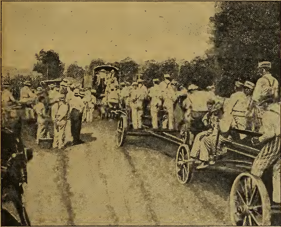
This is one of the many road-grading crews that were so conspicuous in Missouri during the two days of the good roadwork
