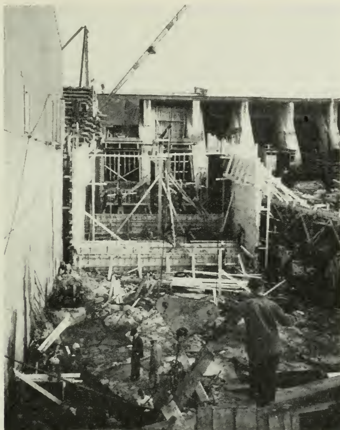
EAR FALLS GENERATING STATION — ENGLISH RIVER Construction work during 1947 on the fourth unit — 5,500-kilowatts (7,500 horsepower)
