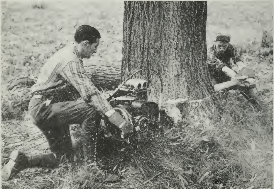
CLEARING THE GROUND Before the dam holds back the river, the areas to be flooded are cleared. The power saw illustrated is a great help in clearing operations
