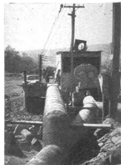
Ventilating Equipment for Supplying Air Tunnel
