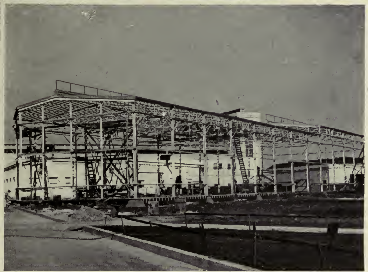
WESTERN AND EASTERN STUDIOS; ABOVE—STAGE PLATFORM IN THE OPEN. BELOW—GLASS-ENCLOSED STUDIO UNDER CONSTRUCTION
