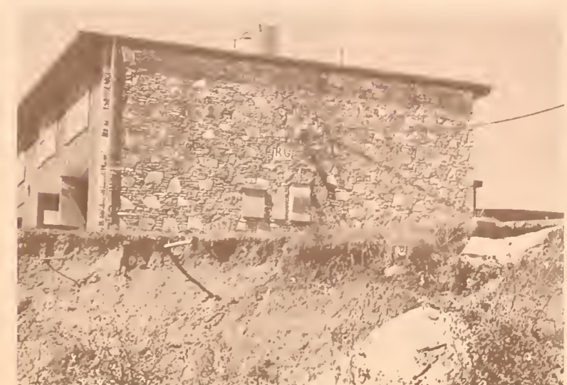
Unprotected soil near this apartment building washed away during heavy rains. The concrete waterway (right) has been damaged and the service pipes (left) are exposed.
